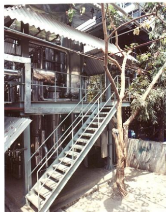
Installation of a triple effect evaporator system at a textile mill in Bombay, India to recover caustic soda chemicals from the wastewater effluent. This resulted in a reduction of 40% of the mills requirement for caustic soda purchases.
