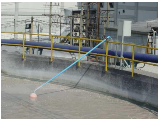
Installation of “dissolved oxygen” measurement system control device leading to increased energy efficiency.
