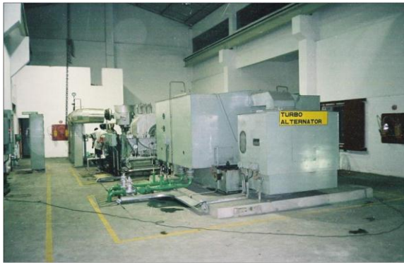
New steam & power generation system in a paper mill
