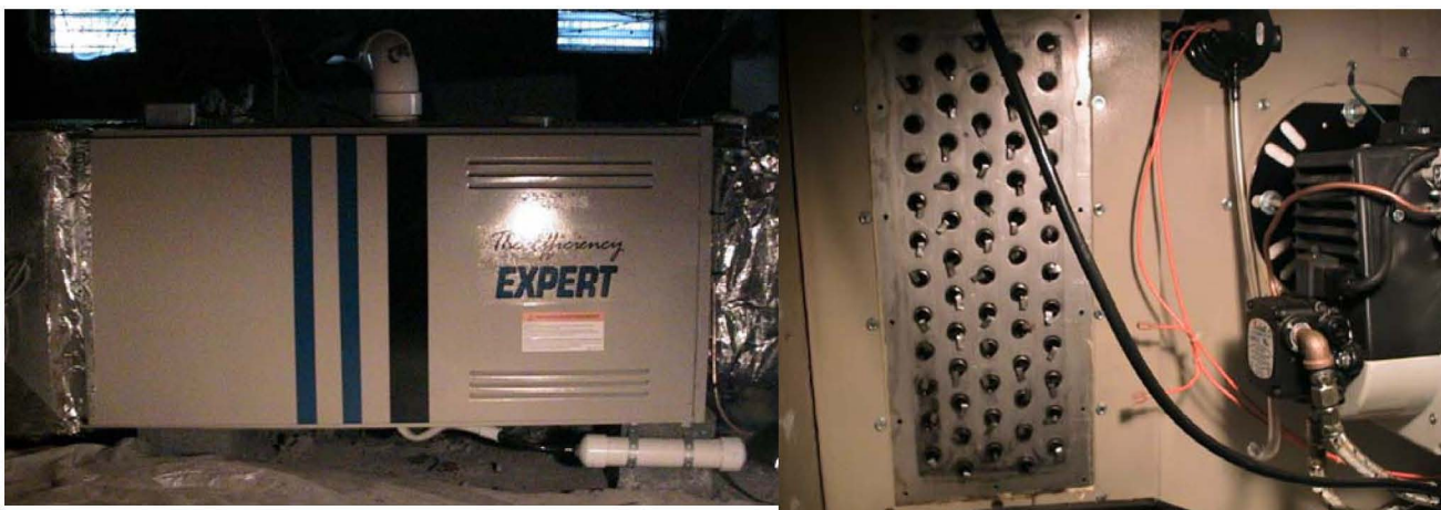
Figure 17 Condensing furnace and heat exchanger from house "B"
