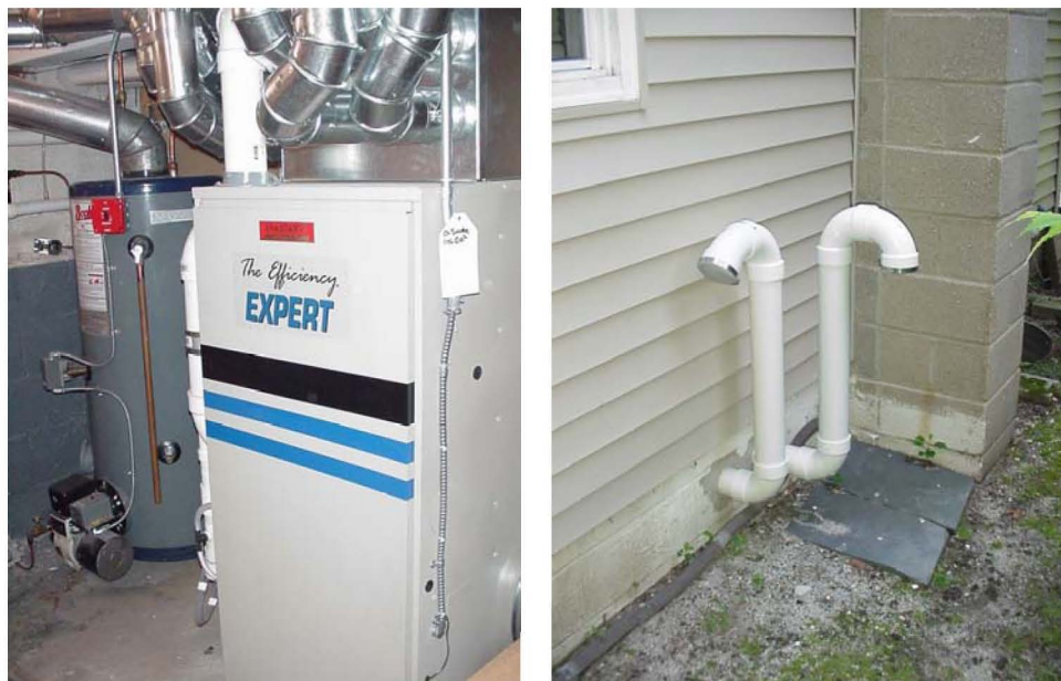
Figure 20. Installed unit and vent arrangement. Site visited early in project. Unit was removed before study was concluded
