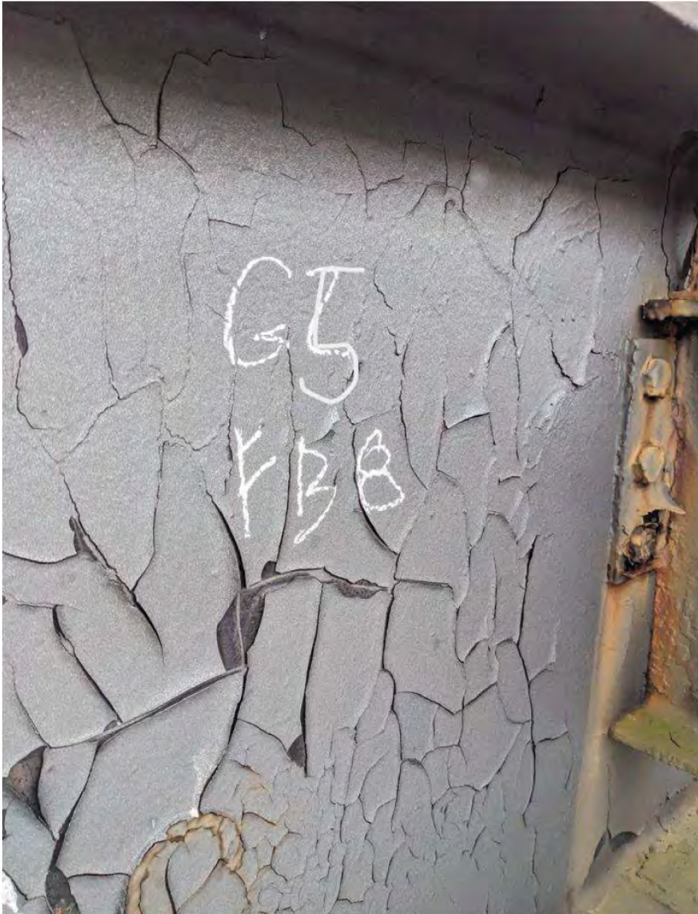
Photo 11: General photo showing the coatings breakdown along the interior side of the girder web. Localized corrosion can be observed in areas where the coatings have broken down further.
