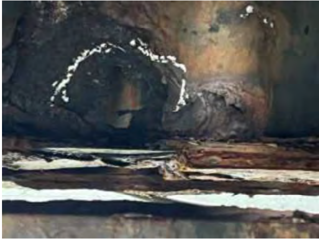
Photo 5 - Full section loss of through the web of joists.
