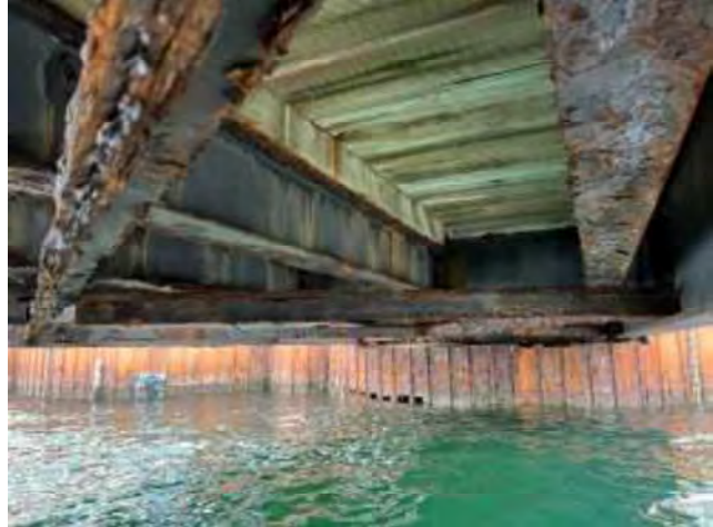
Photo 10 - Braces with severe corrosion damage prior to corroded area being removed.
