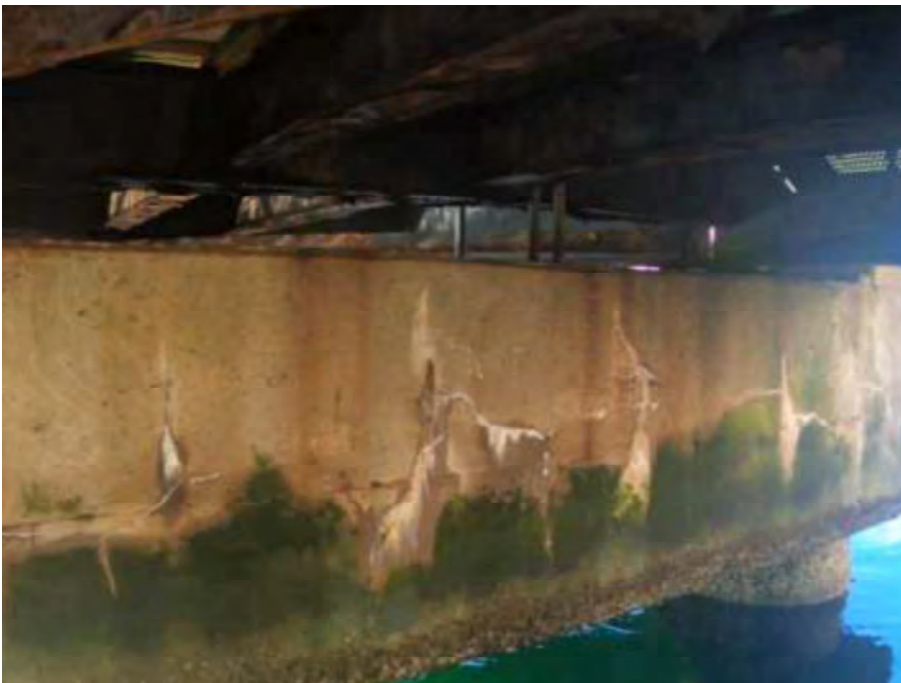
Photo 19 - Presence of efflorescence of observed in pile caps.
