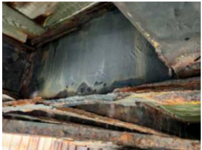
Photo 12 - Beam with full section loss through the flange between the joists.
