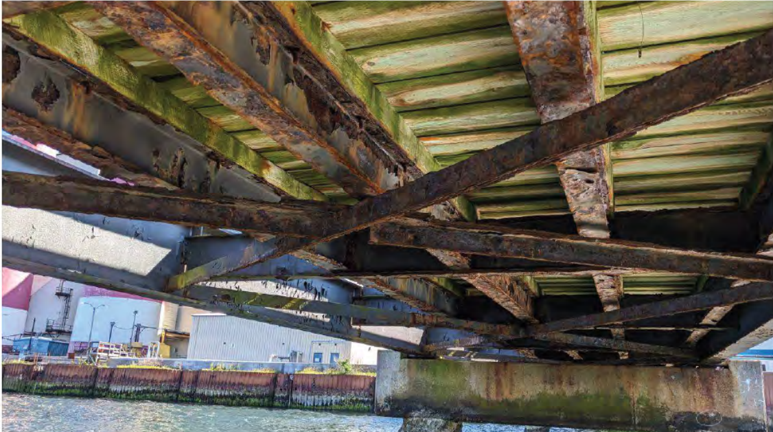
Photo 4: General conditions of the superstructure in Span 3. As can be seen in the photo, the stringers and plan bracing have coatings breakdown in various areas over the length of the members. Corrosion is visible, with areas of delamination and flaking steel.
