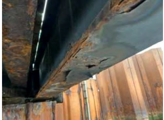
Photo 2 - South Girder at Span A showing corrosion on the flange and coating failure.
