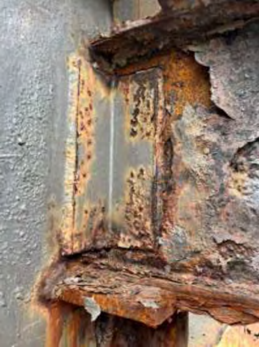
Photo 26 - Connection different from the rest of the structure (South side of North girder on Span A).
