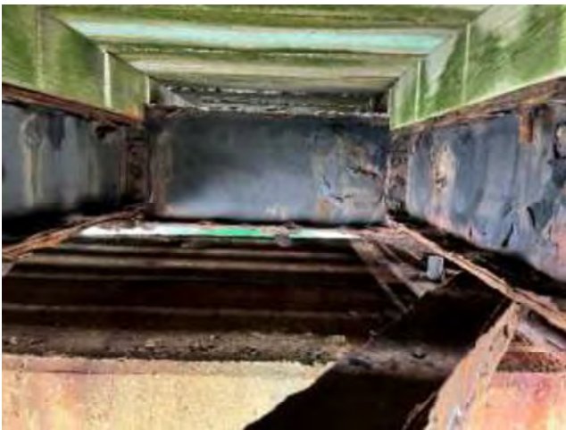
Photo 11 - Beam with corrosion damage.
