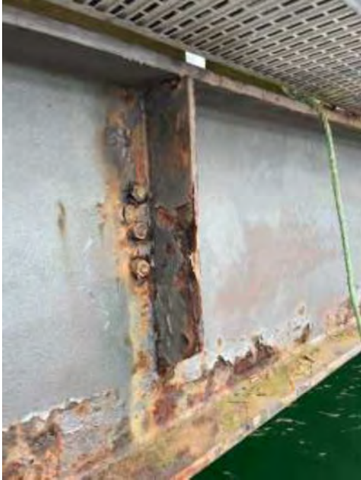
Photo 17 - North Girder at Span C in fair condition with minimal section loss due to corrosion.
