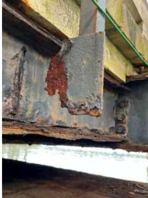
Photo 21 - Full section loss of North handrail to the structure.
