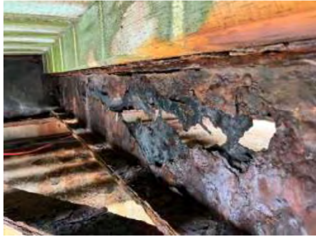
Photo 6 - 2 full section loss through web of joists measuring 18" in total length.
