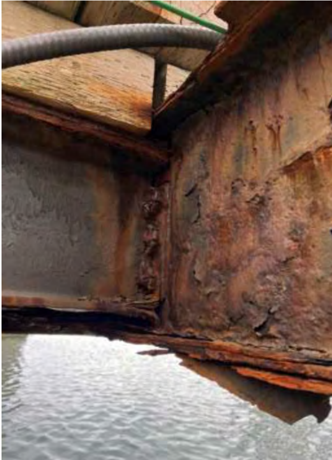
Photo 24 - Poor condition observed in connection at multiple locations.
