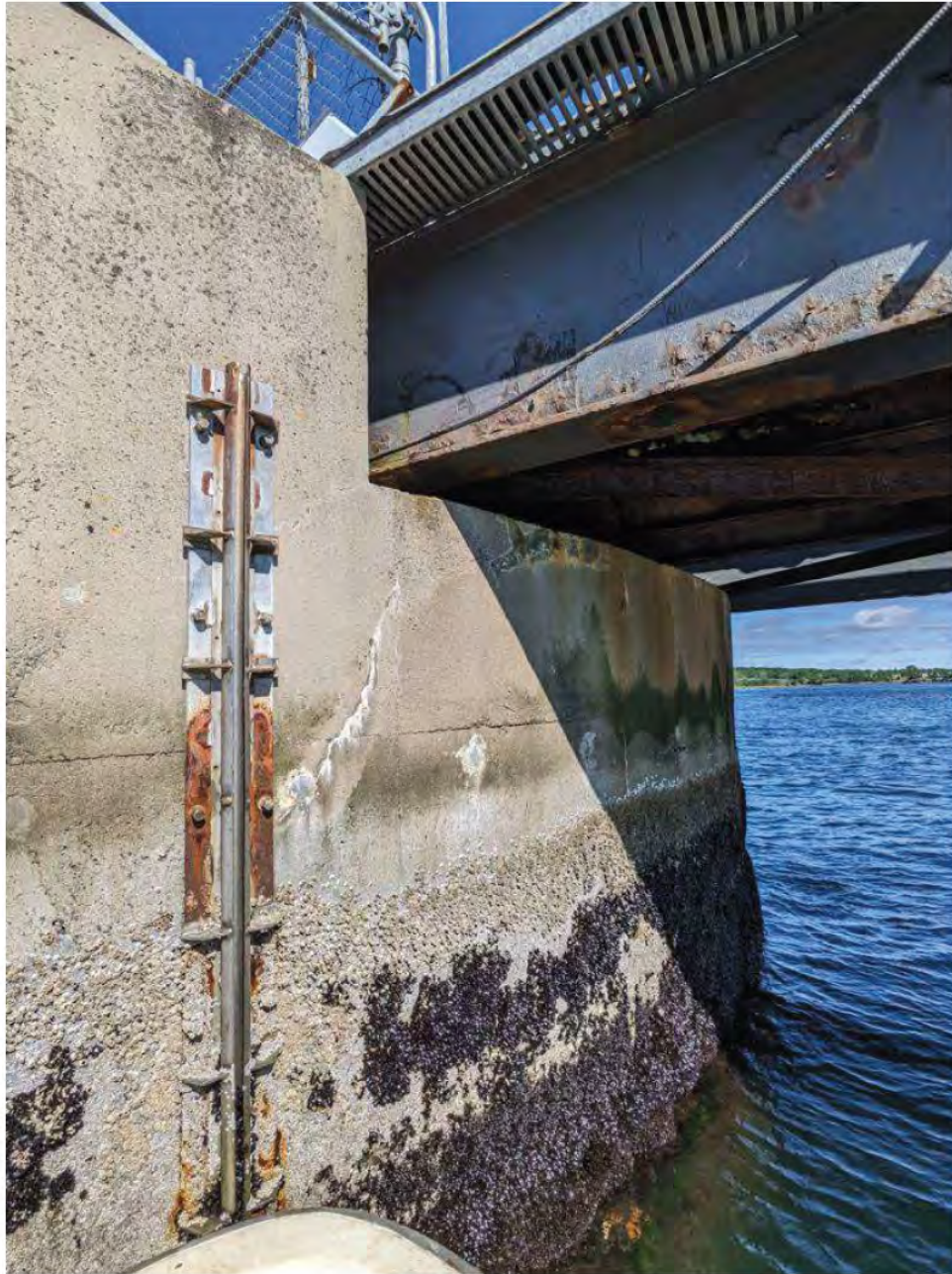
Photo 21: Photo showing the manifold cell structure. Marine growth was observed above the water level at the time of the inspection. There were local cracks and efflorescence visible along the structure.
