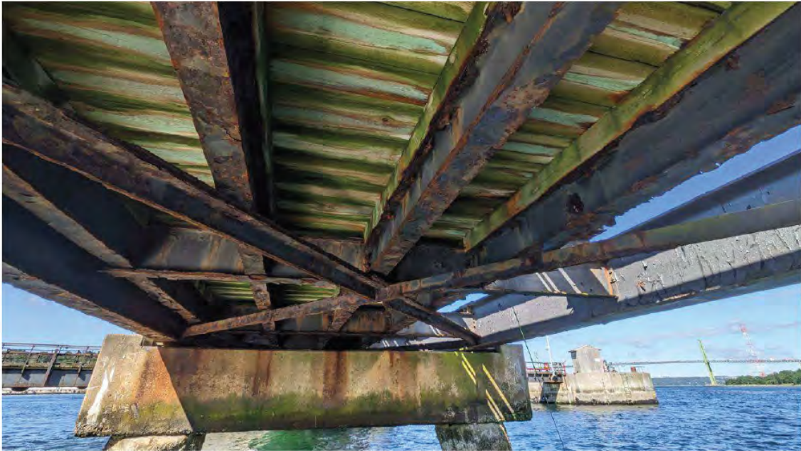
Photo 3: General condition of the superstructure in Span 2. As can be seen in the photo, the stringers and plan bracing have coatings breakdown in various areas over the length of the members. Corrosion is visible, with areas of delamination and flaking steel.
