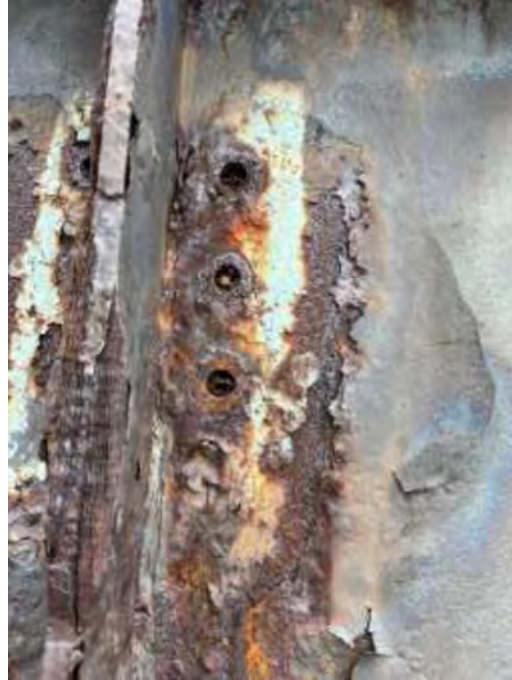
Photo 27 - Connection different from the rest of the structure (North side of North girder on Span A).
