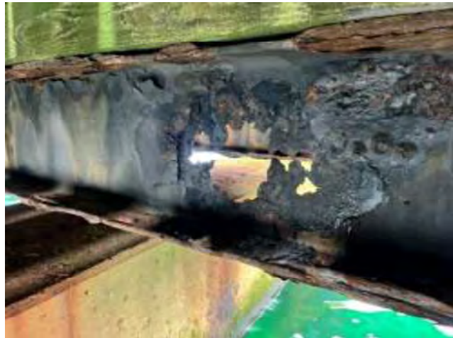
Photo 8 - Full section loss at web of joist extend through the full height of the web and significant section loss in flange.
