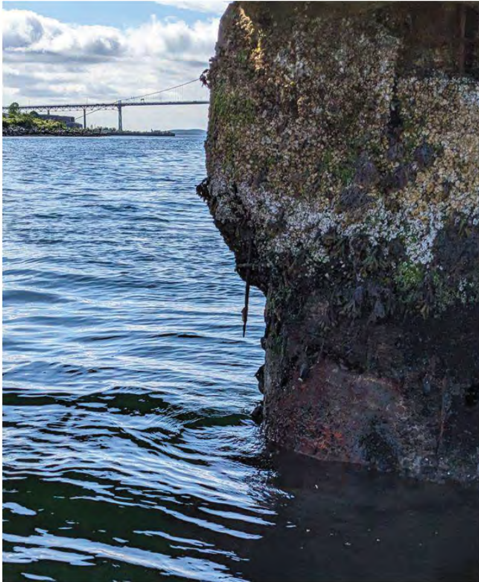
Photo 19: Photo showing the one of the piles at Pier 2. The concrete cover for the steel pile has spalled off locally and the rebar is exposed, and several bars have fully corroded through. The exposed steel pile has started to show signs of corrosion.
