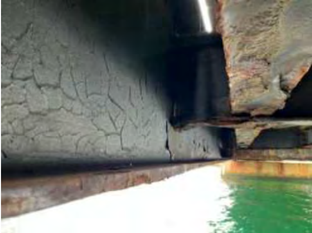
Photo 13 - Coating on girder alligatoring (South girder).
