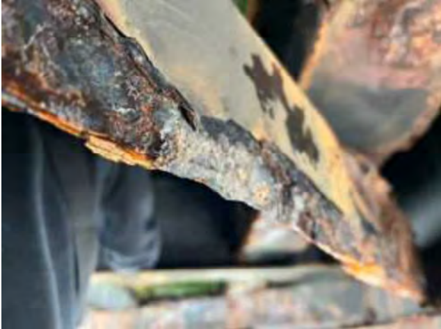
Photo 9 - Braces with severe corrosion damage.
