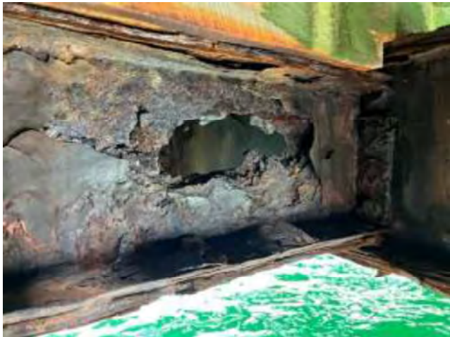
Photo 7 - Full section loss at web of joist measuring 6" long.
