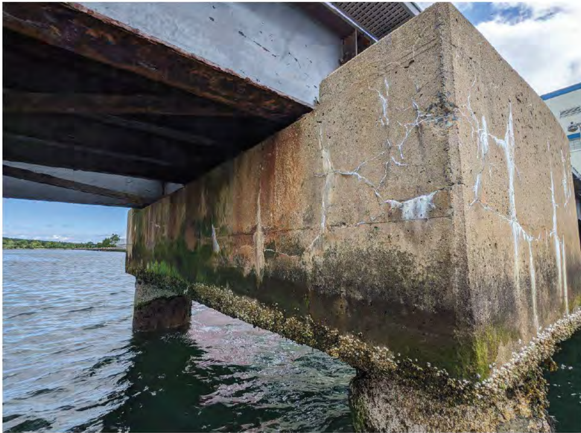
Photo 16: Photo showing the condition of pile cap at Pier 1. Visible cracking throughout the pier cap can be seen, as well as efflorescence.
