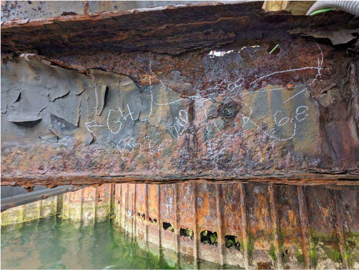
Figure 1: Full Section Loss in Web of FB2
