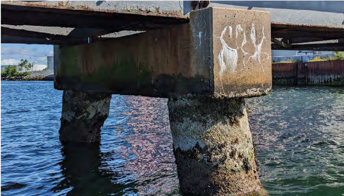
Photo 18: Photo showing the condition of pile cap at Pier 2. Visible cracking throughout the pier cap can be seen, as well as efflorescence.
