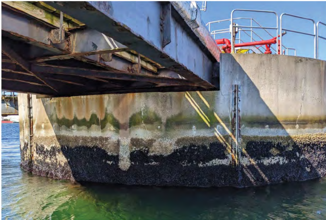
Photo 20: Photo showing the manifold cell structure. Marine growth was observed above the water level at the time of the inspection.
