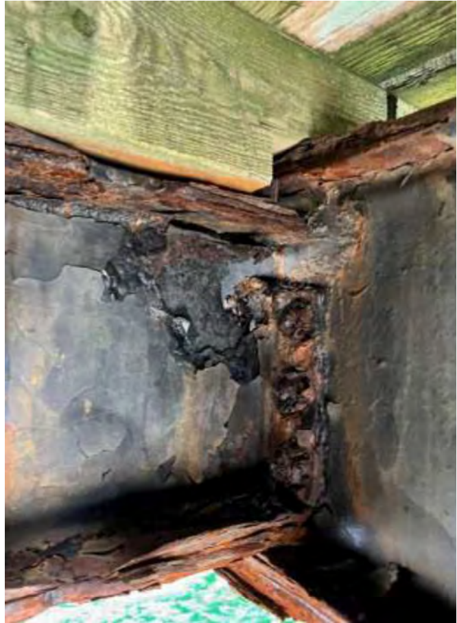
Photo 25 - Poor condition observed in connection at joist to beam connection.
