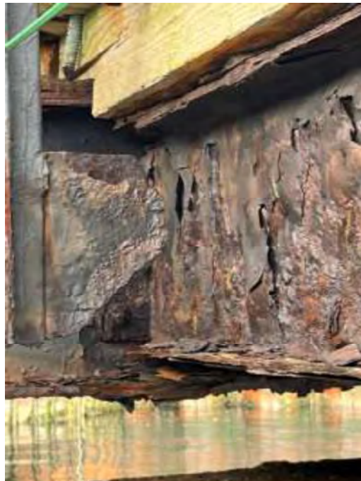
Photo 23 - Full section loss of North handrail to the structure.
