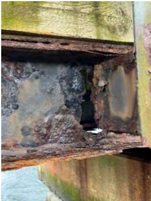
Photo 22 - Full section loss of North handrail to the structure.
