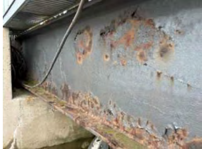
Photo 14 - Coating of girder cracking and rusting (North girder).
