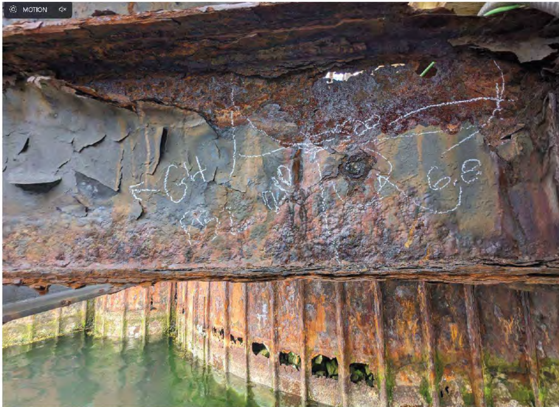
Photo 13: Photo showing the condition of Floor Beam 2. As can be seen in the photo above, a hole has developed in the web of the beam, and both the top and bottom flanges are heavily corroded.
