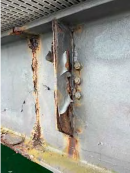
Photo 30 - Coating failure and superficial corrosion observed at the welds at splice location in the girders and the girder bearing plate.
