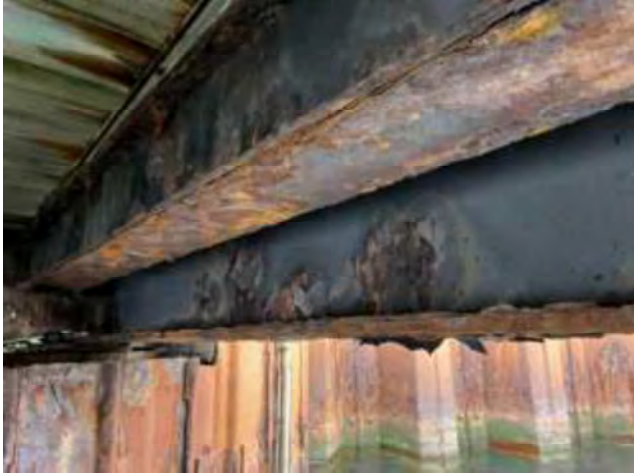
Photo 1 - South Girder at Span A showing localized corrosion in the web.
