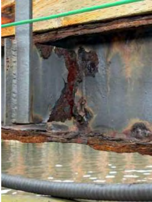
Photo 20 - Full section loss of North handrail to the structure.
