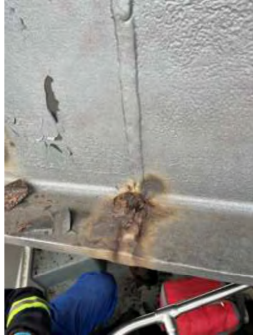
Photo 31 - Coating failure and superficial corrosion observed at the welds at splice location in the girders.
