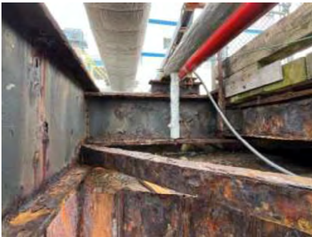
Photo 3 - North Girder at Span A showing corrosion on the flange and web with coating failure.
