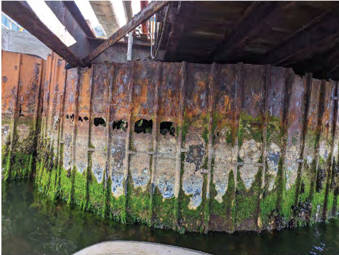
Photo 15: Photo showing the condition of Shore-side Cell. As can be seen in the photo above, there is marine growth over the wetted area of the steel sheet pile wall. There are no signs of coatings, corrosion is visible throughout, with areas of delamination in the steel sheet pile, and full section loss at locations.
