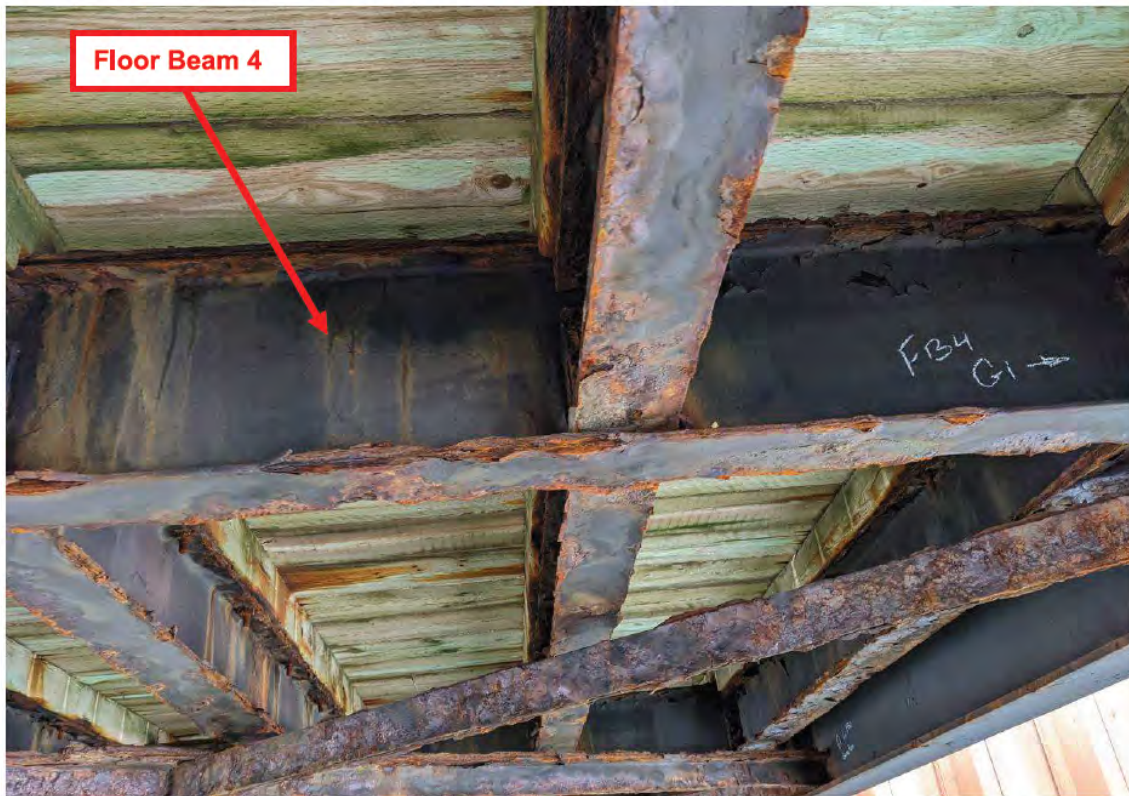
Photo 12: Photo showing the general floor beam condition. Overall conditions are similar between spans. General coatings breakdown, general corrosion observed, both flanges starting to delaminate locally in locations.
