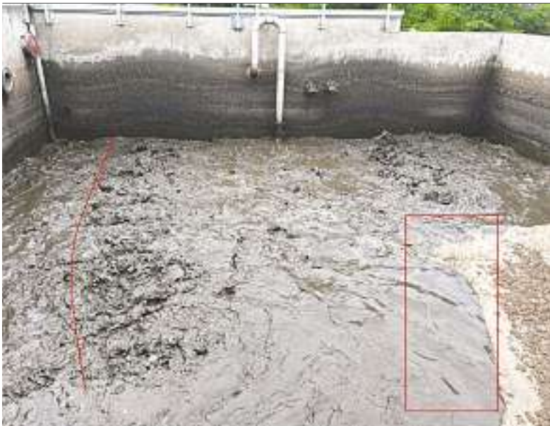
Todd Richard, the director of West Hants’ public works department, showed this image to council Sept. 9 while describing the issue currently plaguing the Falmouth Wastewater Treatment Plant. SUPPLIED
