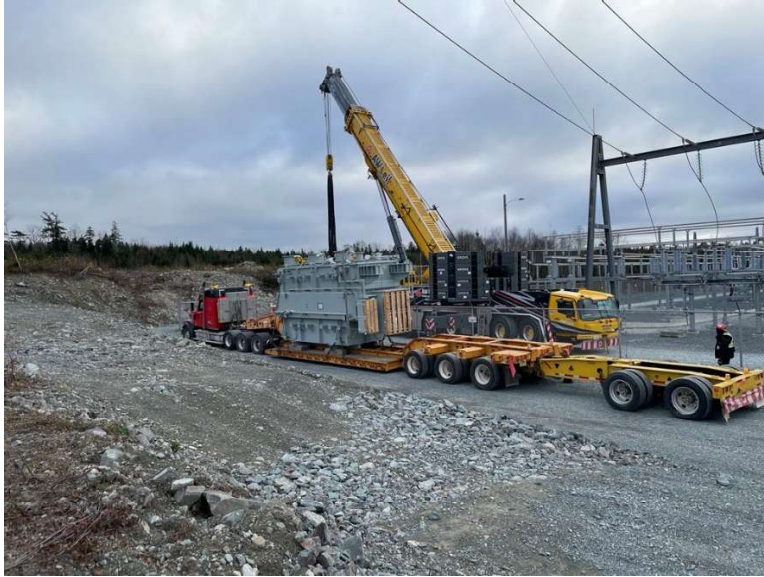
Figure 6 – Main transformer installation for Spider Lake BESS site.
