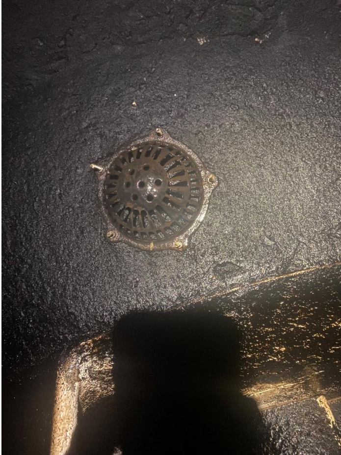
Photo 11: Cooling water screen
