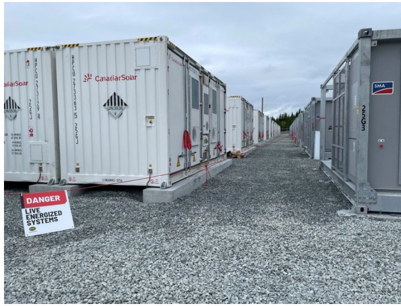
Figure 2: Spider Lake BESS photo showing insulating gravel at grade with row of battery enclosures on left and row of power conversion systems on the right during warm commissioning activity.
