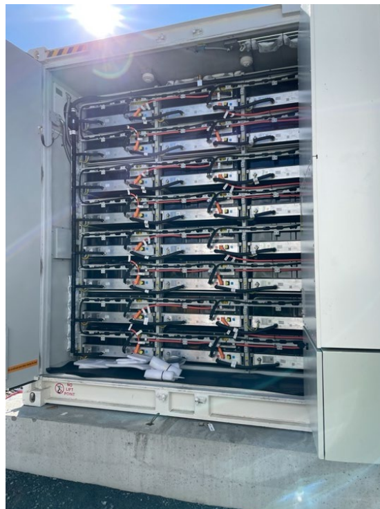
Figure 3: Interior of Battery Enclosure showing three of six racks containing eight individual battery modules per rack.
