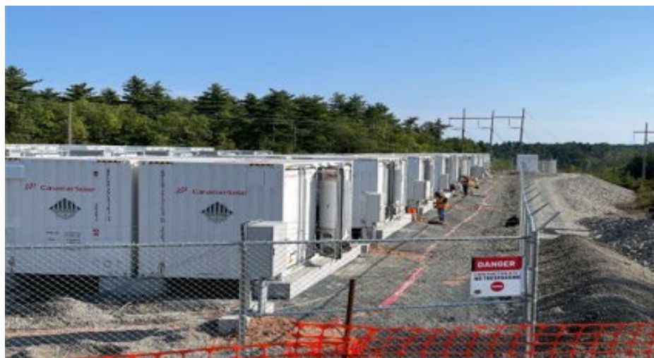
Figure 1: Installed Battery Enclosures at Bridgewater BESS Site.
