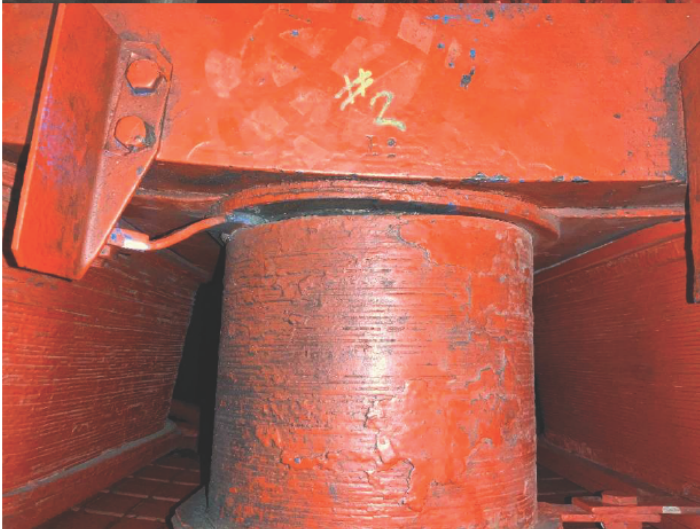
POLE 2: SECTION OF THE COLLAR MISSING.
