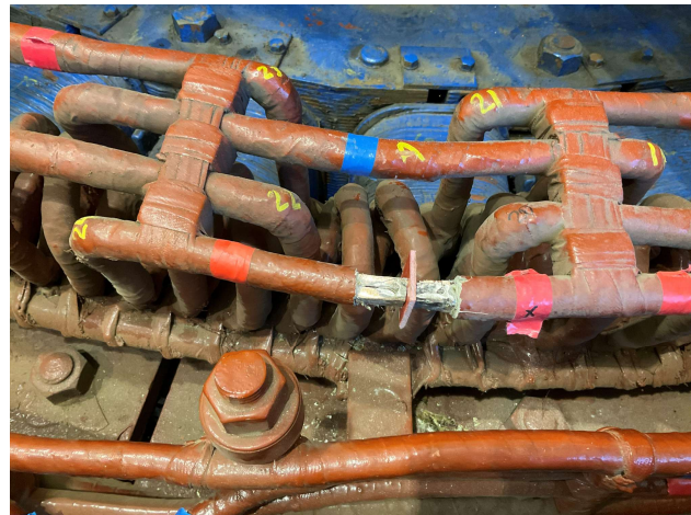
Above picture showing a jumper that would have been cut to isolate a segment of the winding for testing.
