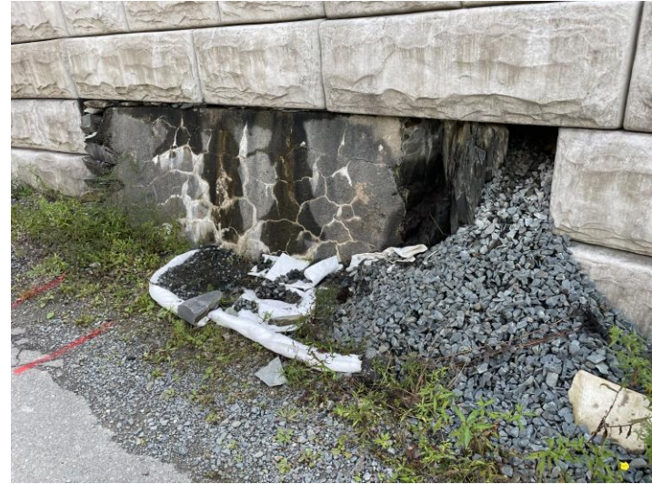
Photo 6: Hydrocarbon impacts in shallow soils/bedrock at base of substation retaining wall. Photo taken on September 11, 2024.
