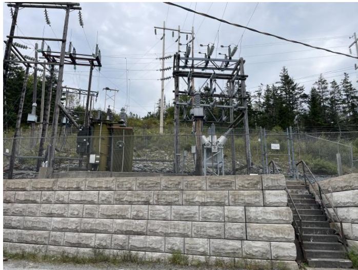
Photo 3: View of transformer substation on north side of the site, looking east. Photo taken on September 11, 2024.
