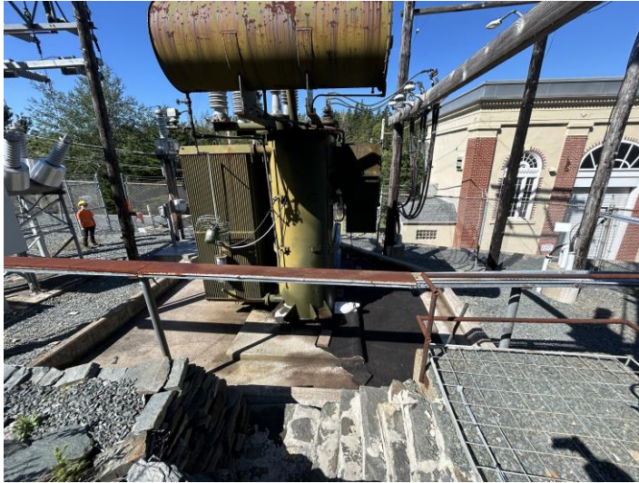
Photo 5: Transformer substation area of release and oil staining on concrete containment floor. Photo taken on August 30, 2024.
