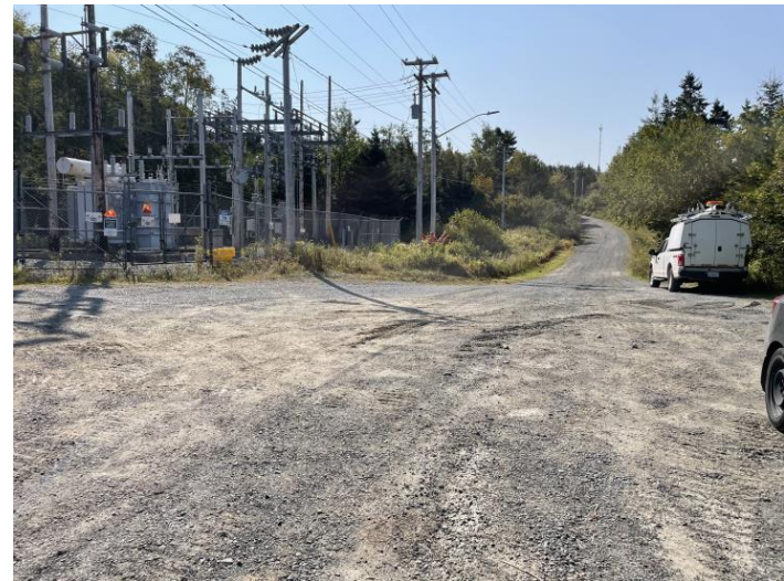
Photo 4: View of transformer substation on south side of the property, looking southeast. Photo taken on September 11, 2024.
