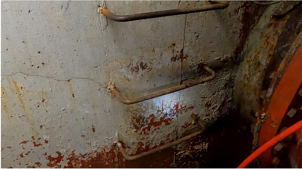
Figure 48: Crack on the South wall
