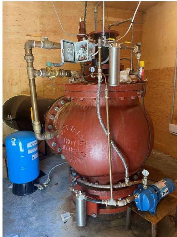
Figure 37: Pressure relief valve
