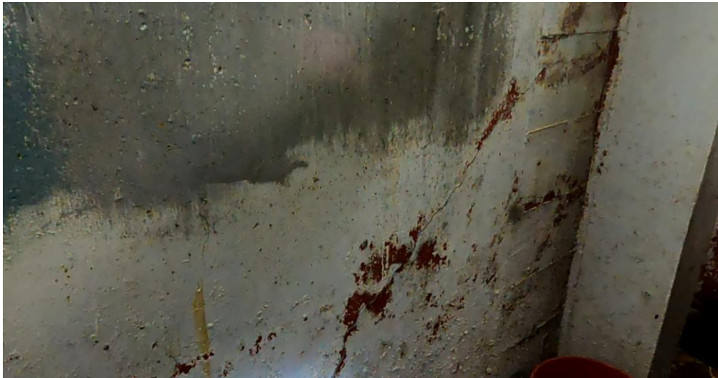
Figure 46: East wall crack
