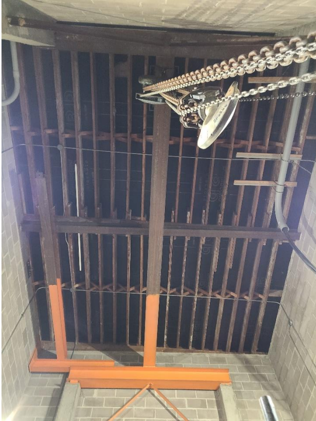
1. Roof framing, hoist beam and chain hoist.
