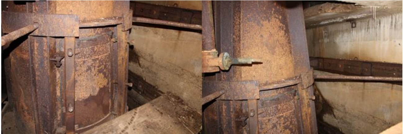
Figure 27: Draft tube exterior, corrosion present, but expected, no damage noticed
