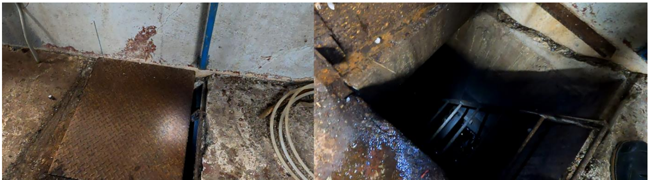
Figure 49: Draft tube access hatch
