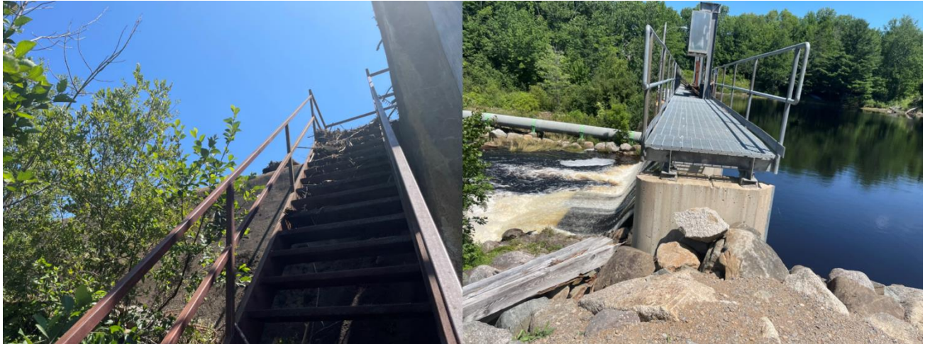
Figure 56: Dam Access points are unsafe
