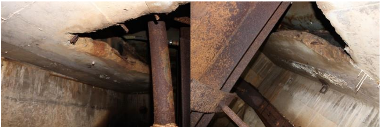
Figure 28: Areas with concrete and rebar exposed
