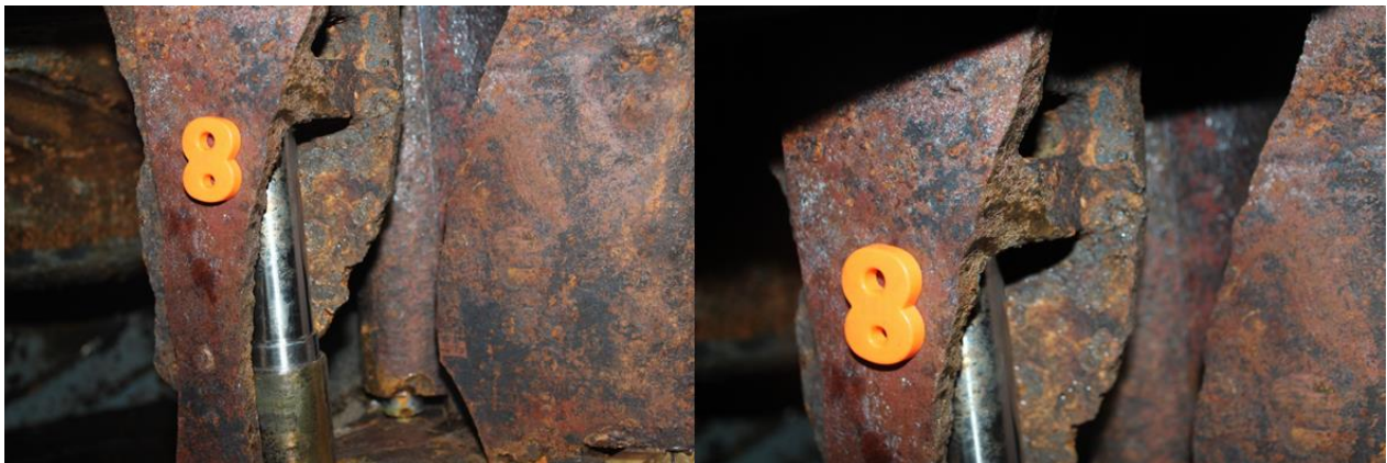
Figure 18: Wicket gate 08, half attached to the pivot shaft
