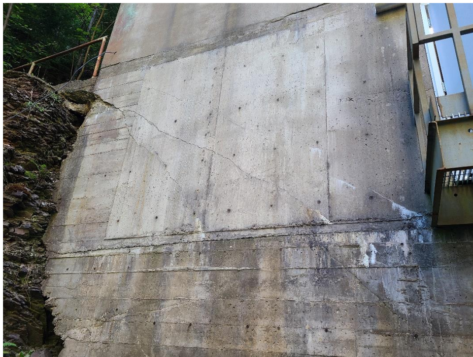
4. Wall cracks from previous photo on the exterior surface of the wall.
