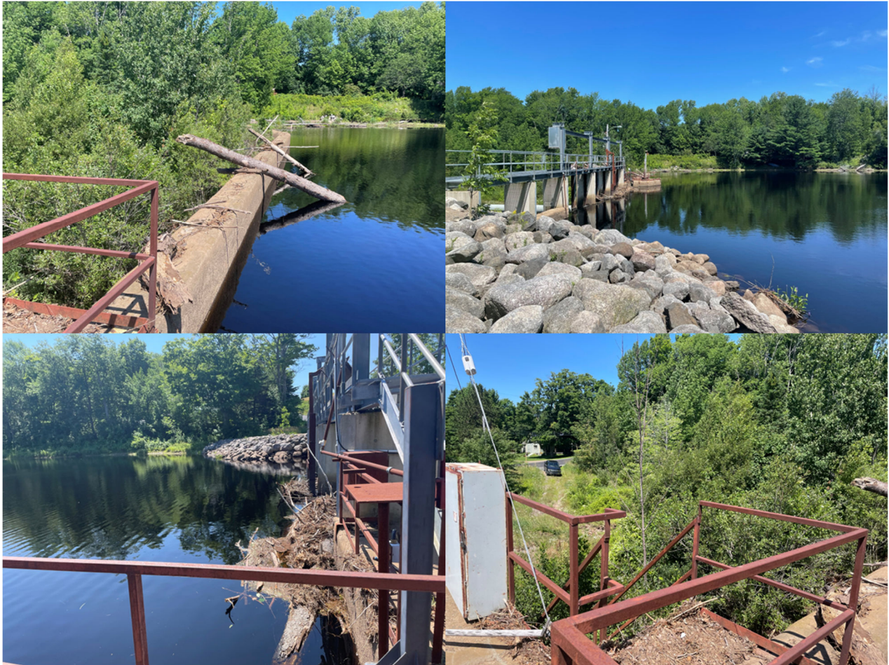
Figure 58: Debris across the dam
