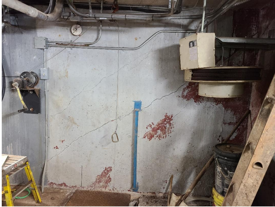
3. Cracks in North concrete wall at intermediate level.
