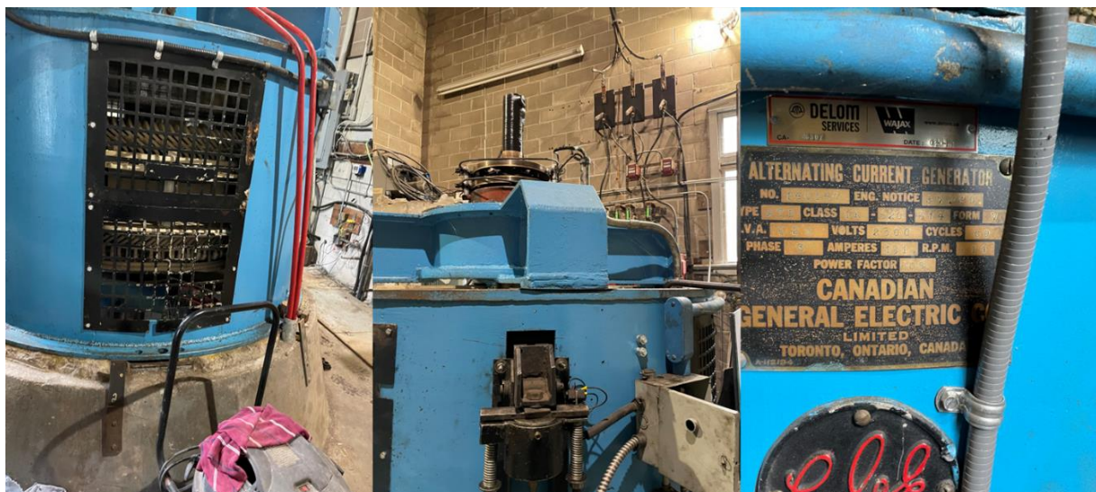
Figure 29: Generator at Factorydale Powerplant
