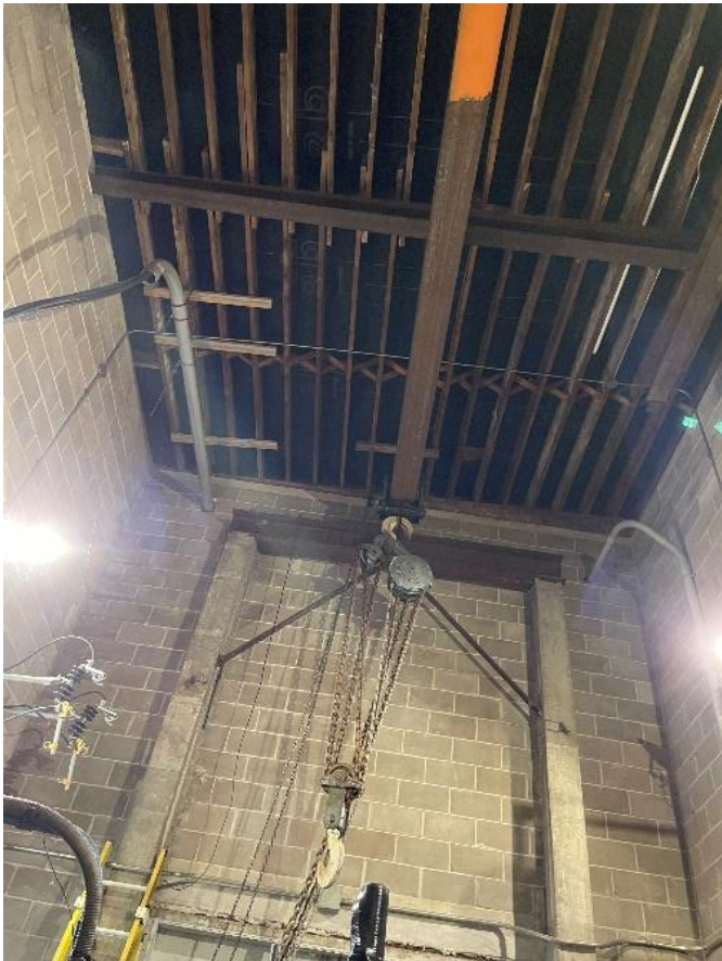
Figure 35: Chain hoist manual crane
