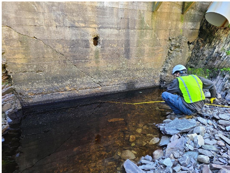
10. Probing undermined area below base slab.
