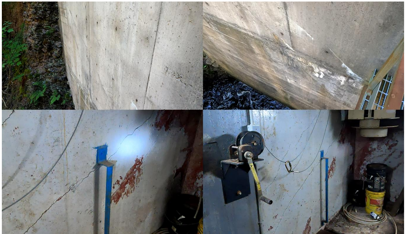
Figure 45: North wall crack
