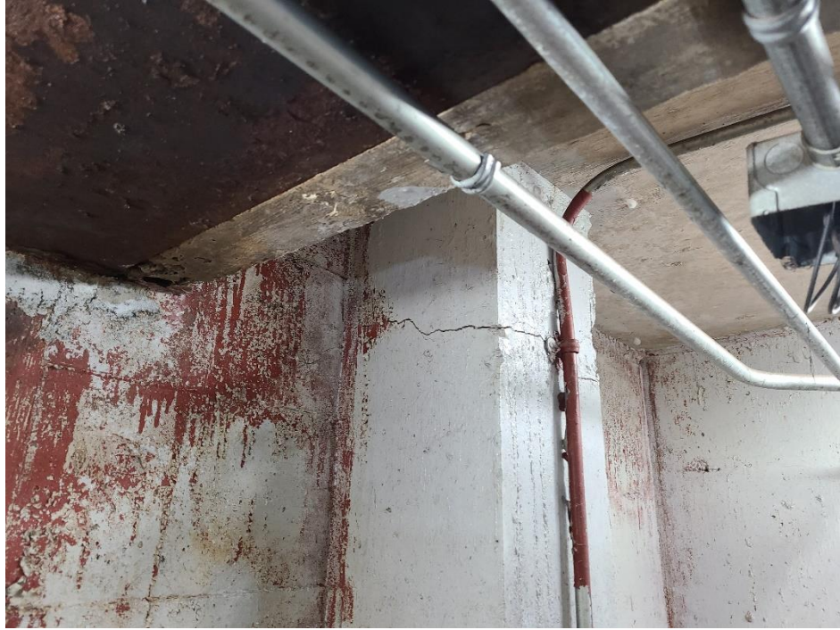
7. Wall cracks shown in previous photo that continue into column.
