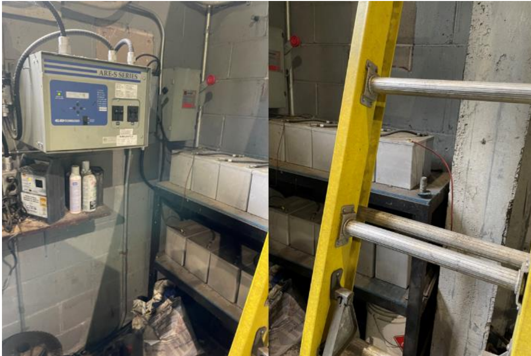
Figure 34: Battery bank and charger
