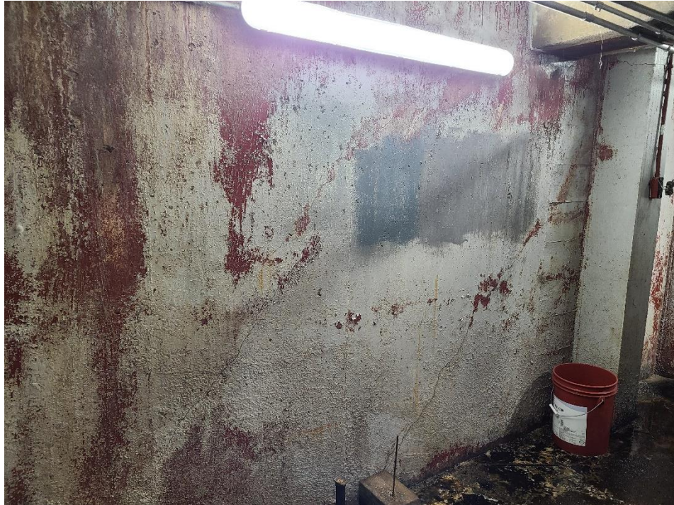
6. Interior cracks on east wall, intermediate level.
