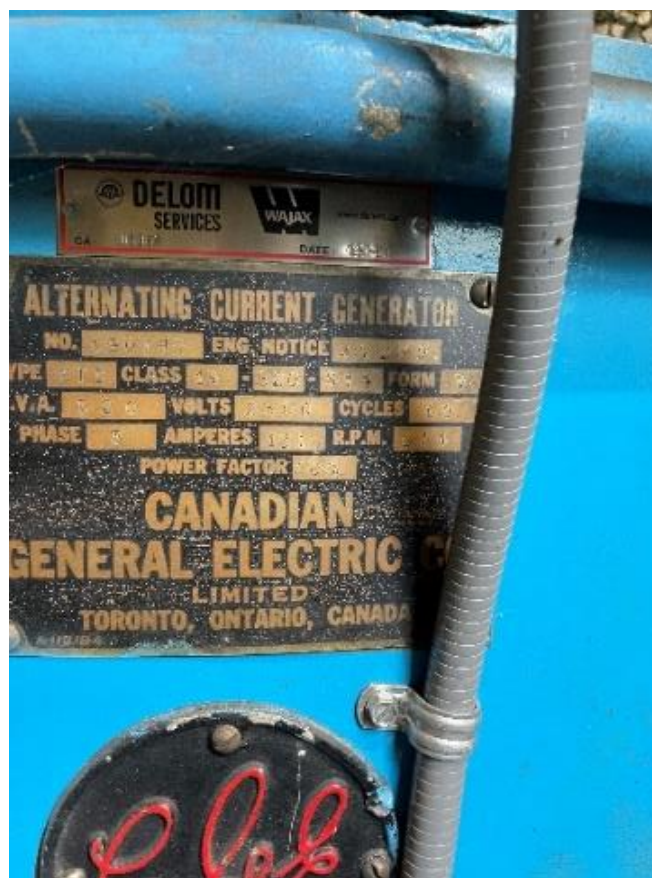
Figure 1: Generator Name Plate
