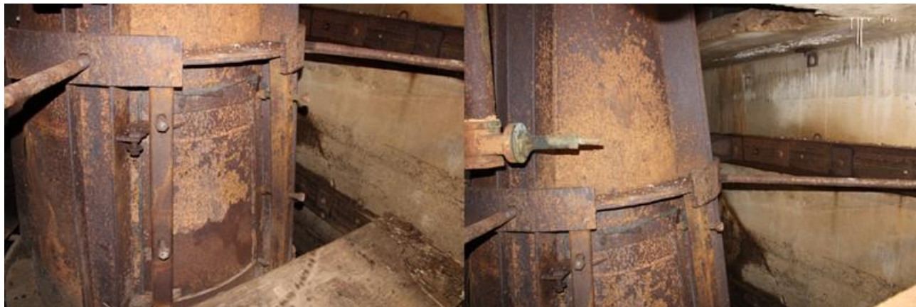
Figure 50: Draft tube exterior, corrosion present, but expected, no damage noticed
