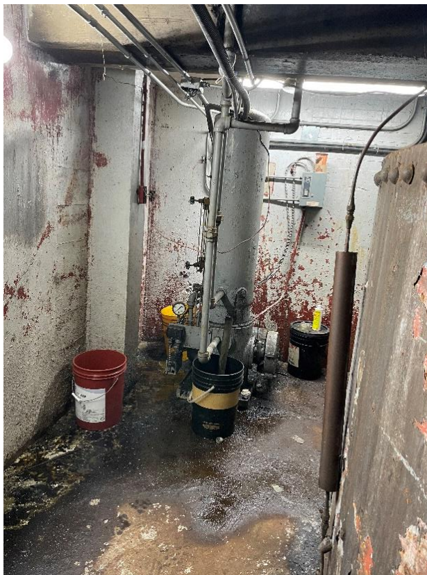
Figure 33: Governor Oil tank, turbine level
