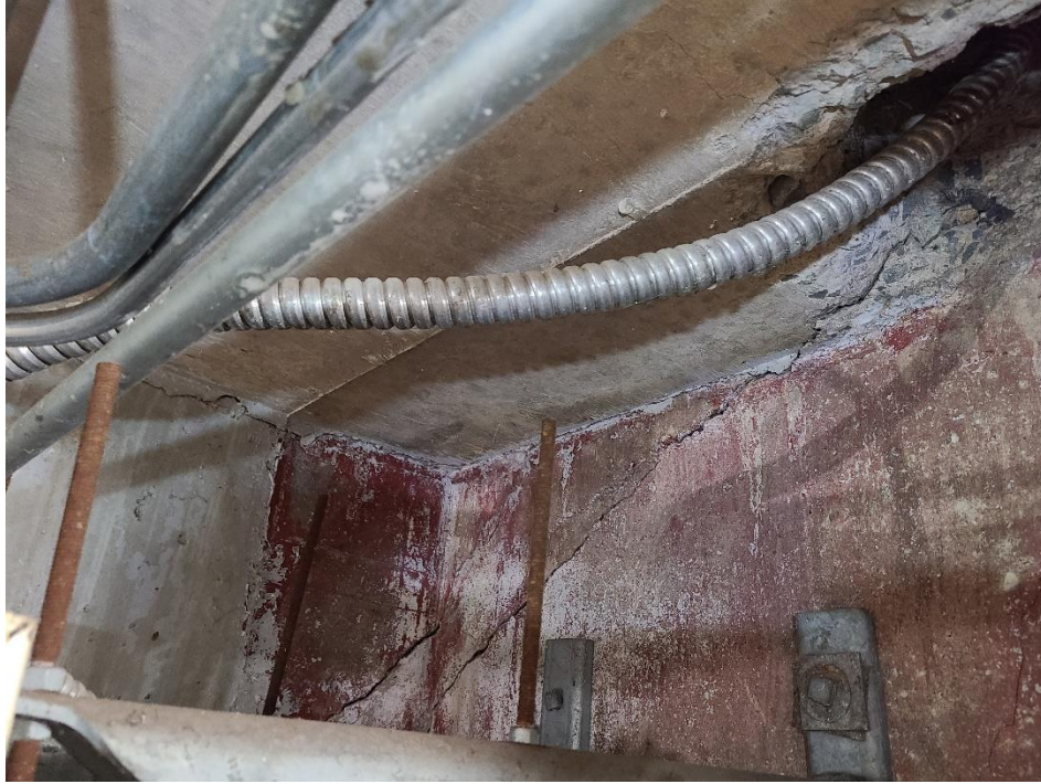
5. Interior wall cracks at northeast corner, Intermediate level.
