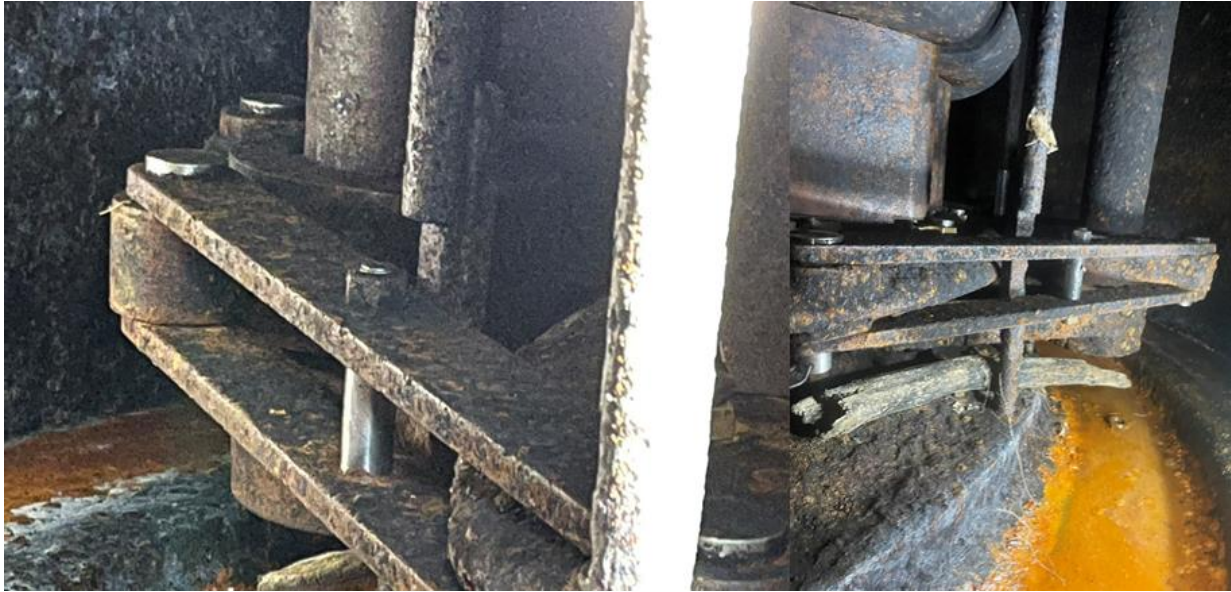
Figure 9: Wicket Gate Mechanism Arms - left and right arms. Notice the wood log on the right picture.
