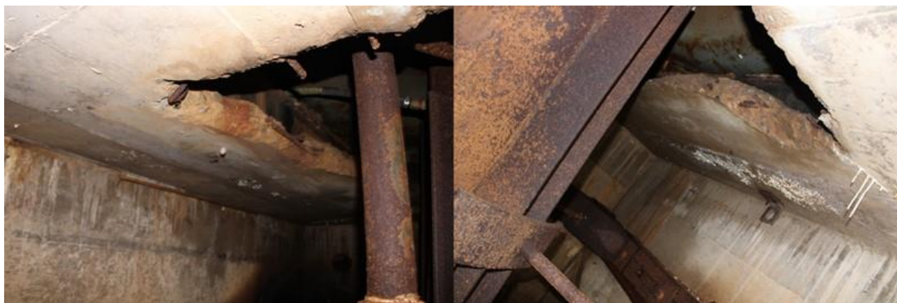
Figure 52: Areas with concrete and rebar exposed
