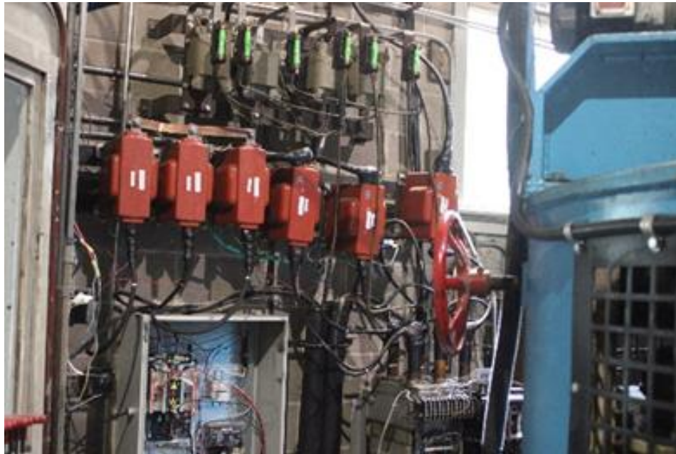
Figure 26: Description of Switchgear.
