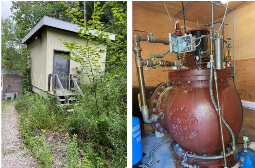
Figure 18: Surge Valve Building and valve.
