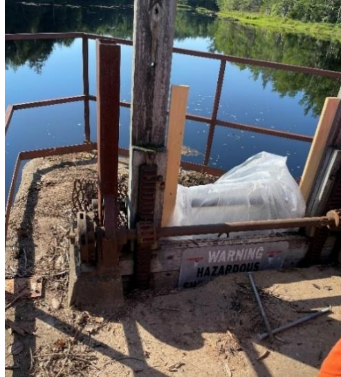
Figure 15: Intake gate in closed position.
