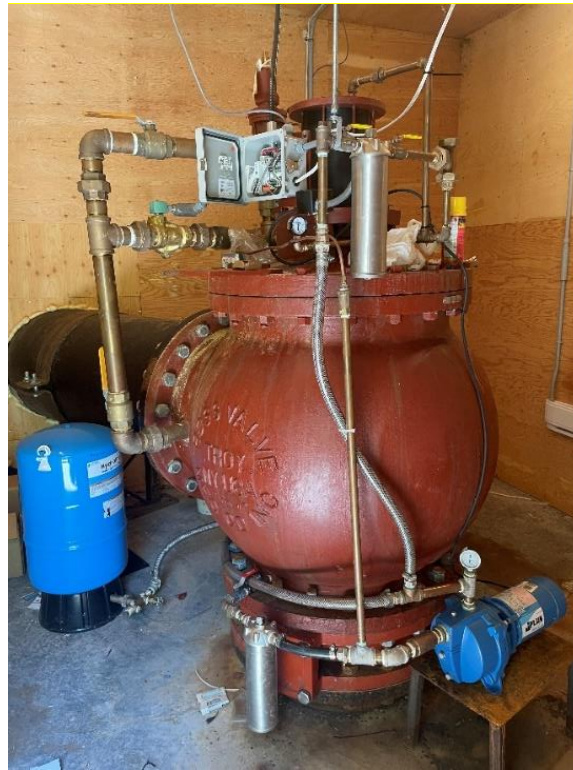
Figure 25: Pressure relief valve.
