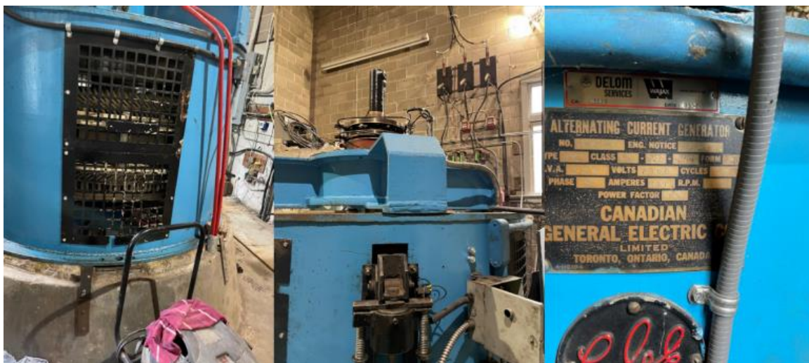
Figure 10: Description of Generator installed.
