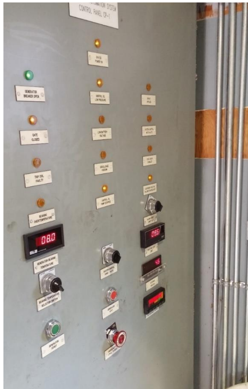
Figure 27: Current panel of the PLC Control and Automation System to be Replaced.
