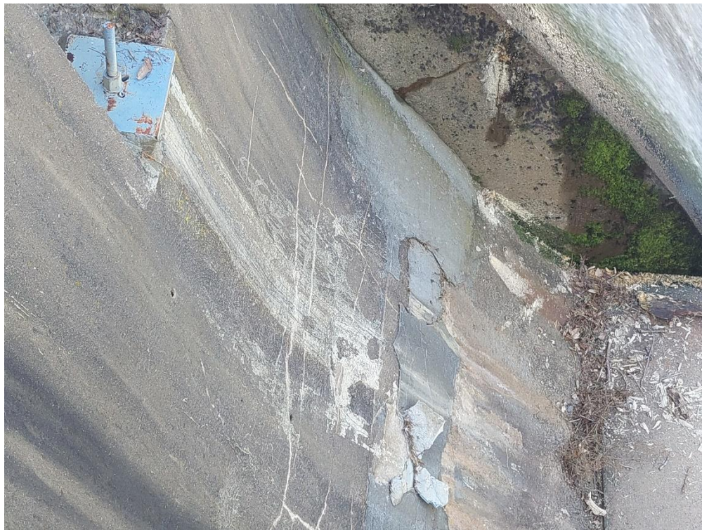
Photo 20 Spalling and Efflorescence Next to Penstock
