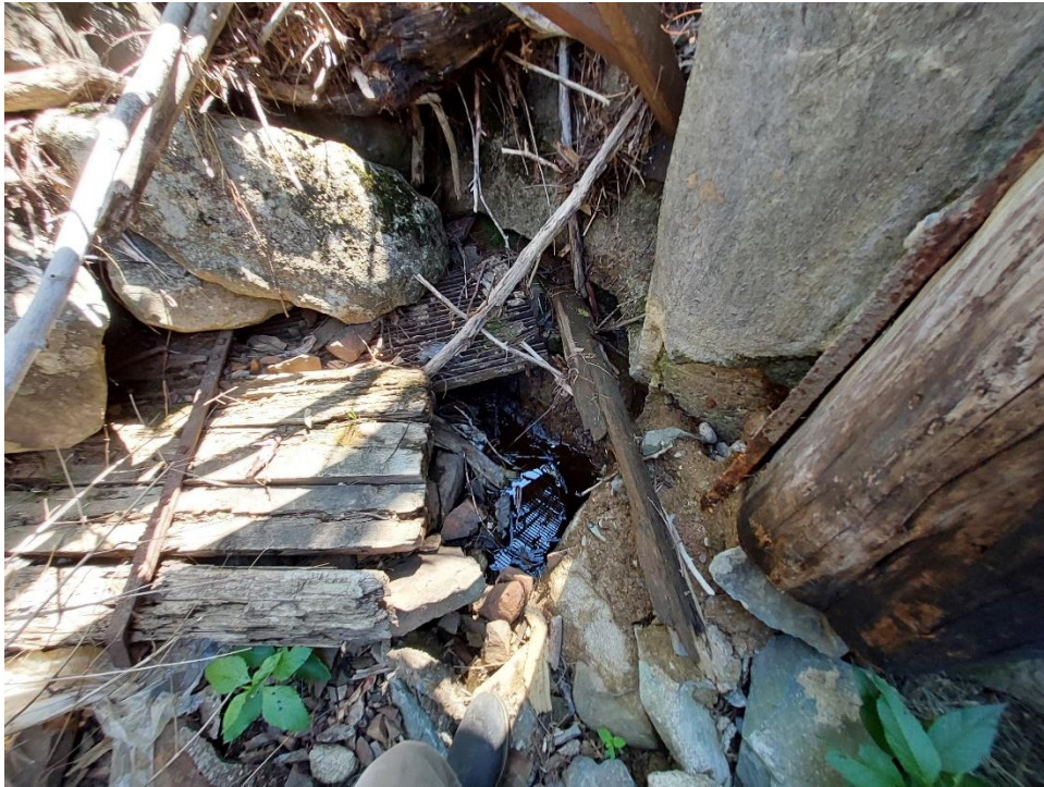
Photo 27 Ponded water and scouring around base of power pole beside Penstock Intake
