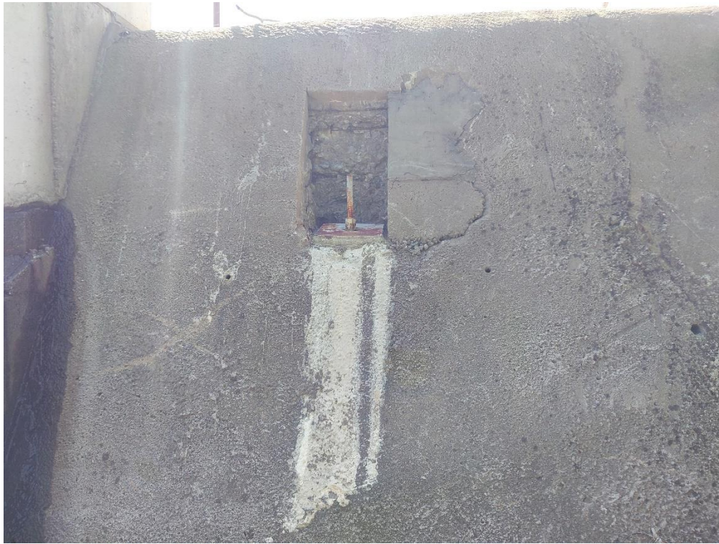
Photo 7 Efflorescence Below Post-Tensioned Anchor at Exposed Portion of Left Dam Section
