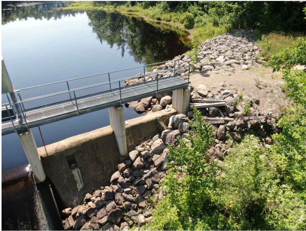
Photo 3 Left Dam Section (Partially Entombed)
