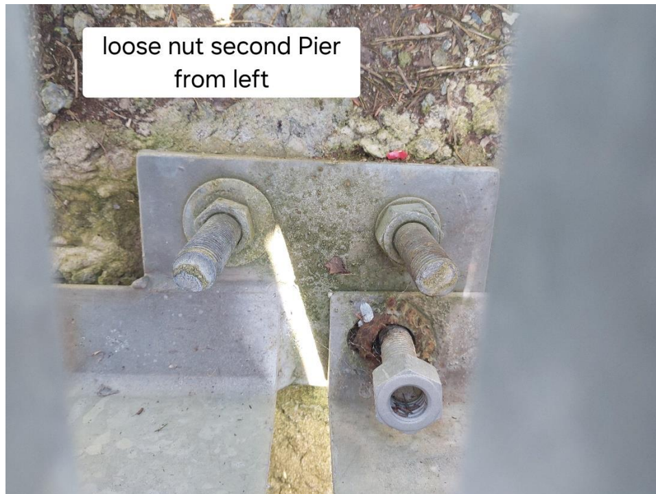
Photo 15 Loose Nut on Catwalk Plate, Second Pier from Left
