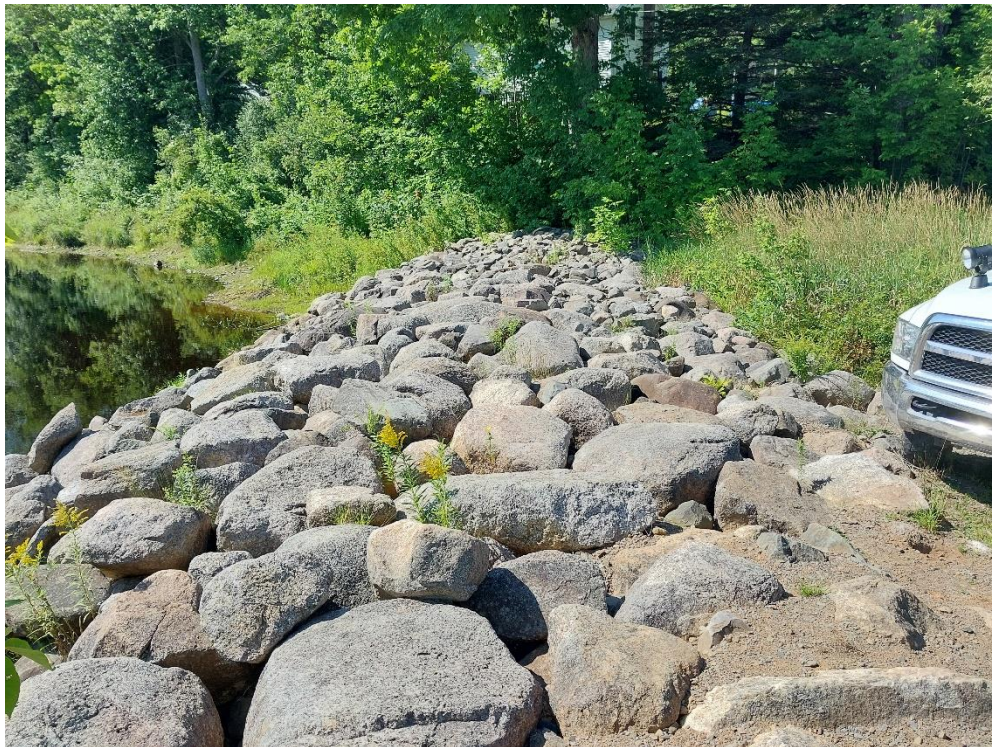
Photo 8 Entombed Portion of Left Dam Section
