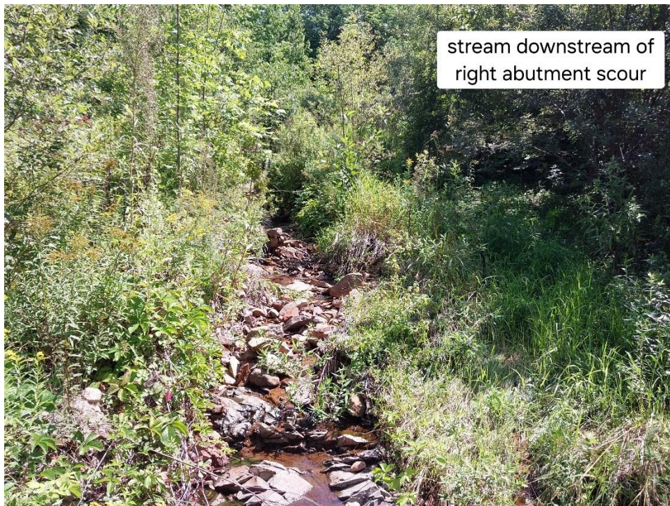
Photo 24 Runoff from Seepage at Right Abutment
