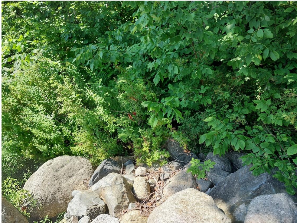
Photo 9 Overgrown Left Abutment
