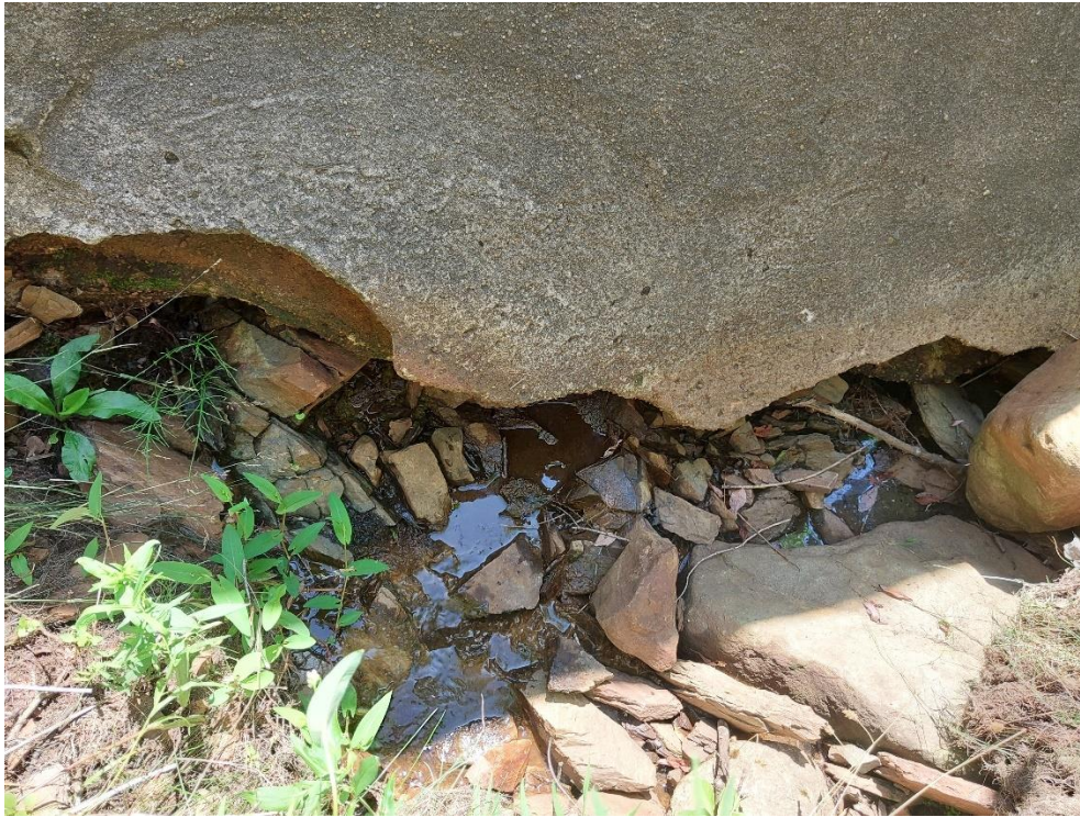
Photo 25 Scour and Trickling water at toe of Right Dam Section
