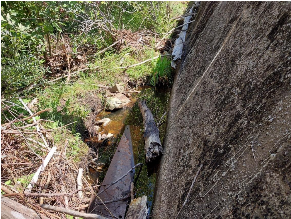
Photo 26 Ponded water at toe of right dam section, next to Penstock intake
