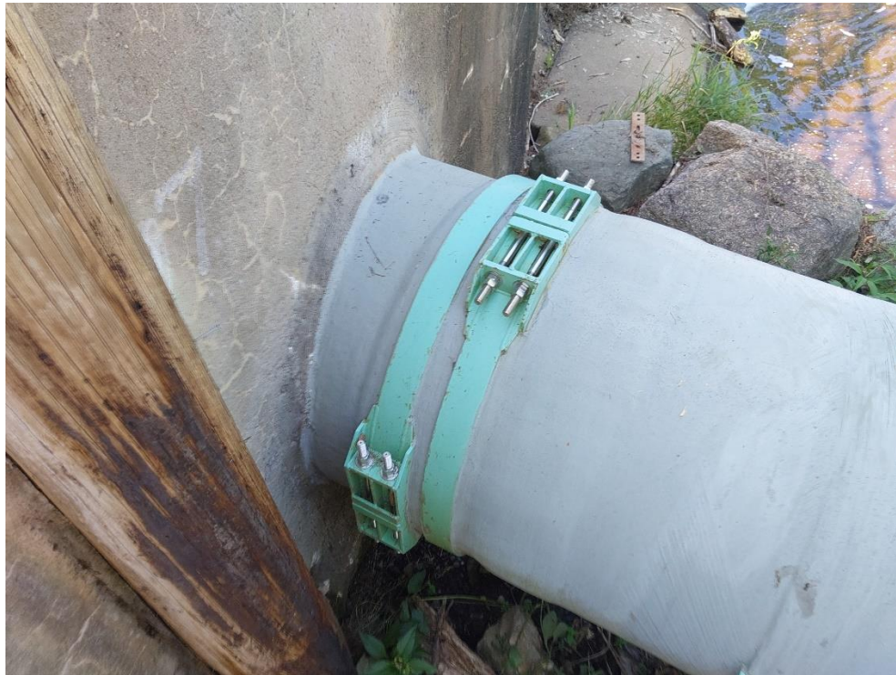
Photo 28 Connection Point for Penstock
