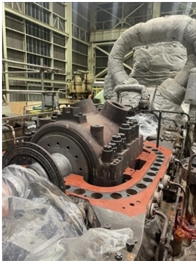
2.2.1.2 AL HP Inner Cylinder Lift
