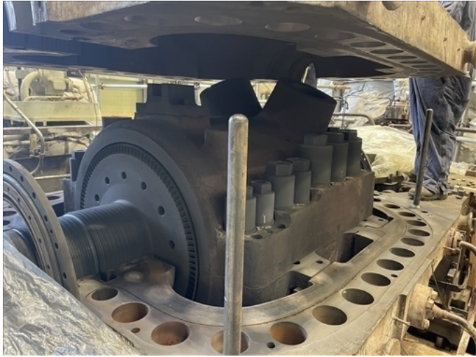
2.1.1.1 AF HP Outer Cylinder Lift
