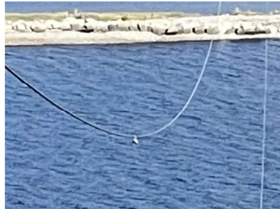
Figure 21 Damper slipped to mid span West circuit, middle phase, from climbing inspection in May 2022. (Figure 3 of August 2023 report)
