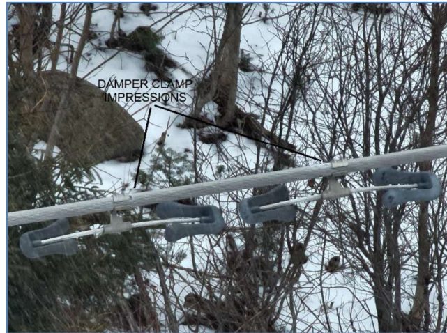
Figure 3 Salvi dampers on the back span on Cape Breton Island showing impressions of previous damper clamp positions, or possible slippage. Detail from Photo No. DJI_20240118000143_0026_Z.jpg
