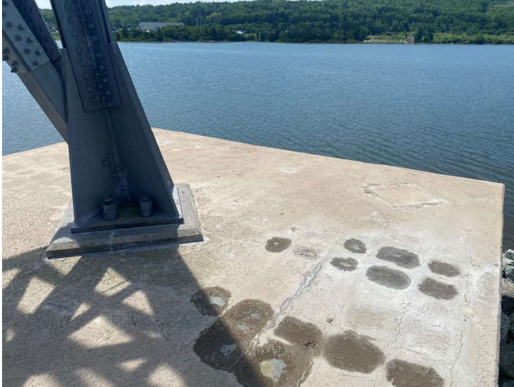
Figure 1 - Str 730, NW foundation, cracking in square pattern
