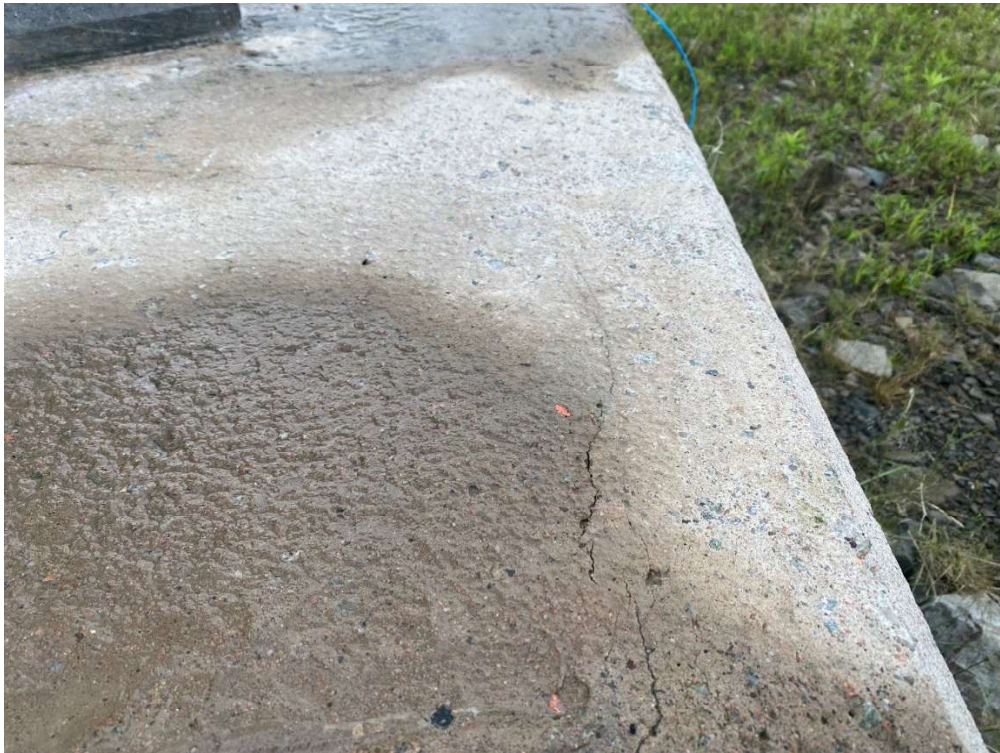
Figure 2 - Str 731, NE foundation, cracking in square pattern
