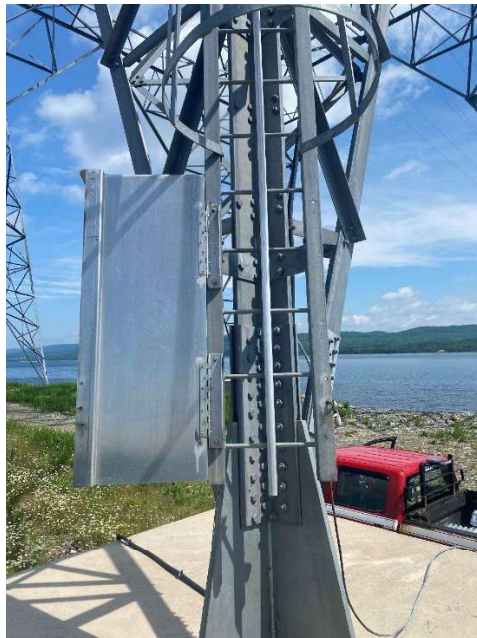
Figure 5 - Str 730, bolts requiring retorquing behind door panel
