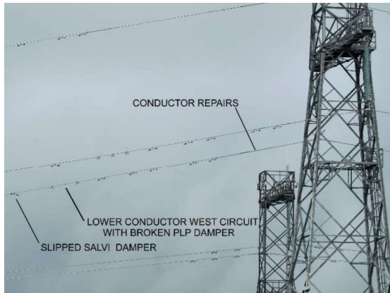
Figure 6 Closer view of bottom phases on crossing side of the suspension structure on Cape Breton Island looking west along the strait. Photo includes the slipped Salvi and broken PLP dampers. Repair sleeves can be seen between the array of dampers and the suspension clamp. Detail from photo No. DJI_20240117231347_0033_Z.jpg
