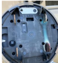
Meter overheated due to socket problem
