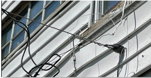
Secondary tap – safety and fire hazard
