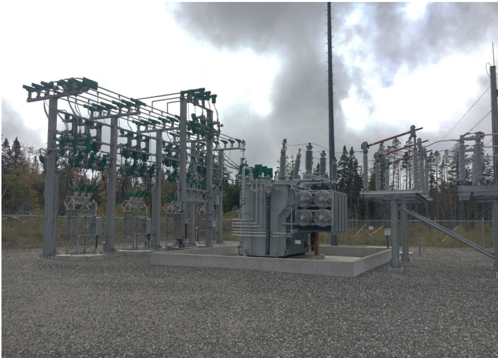
111S - Prime Brook (138kV – 12.5kV)
