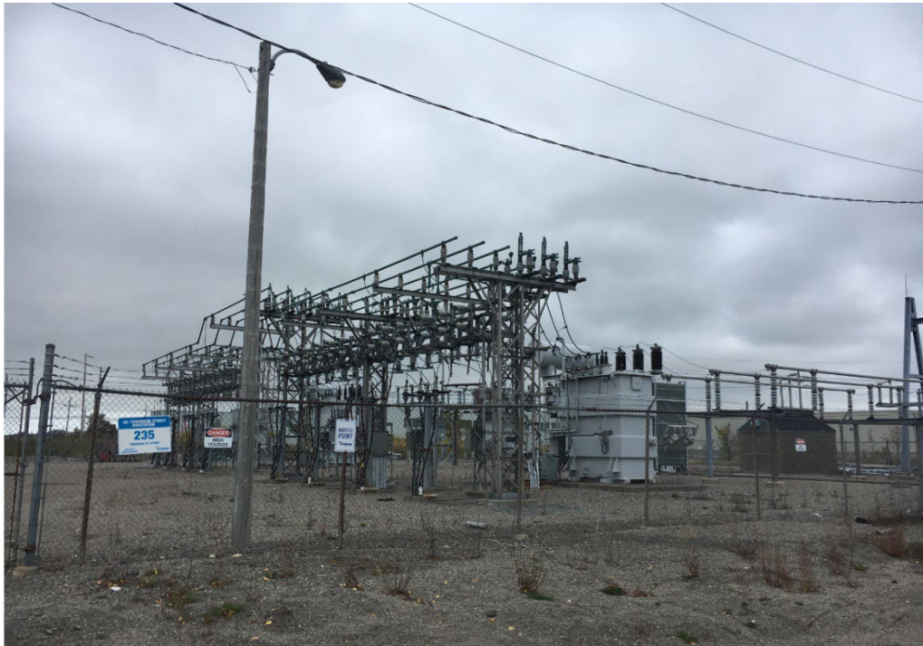
4S – Townsend Street (69kV – 12.5kV)
