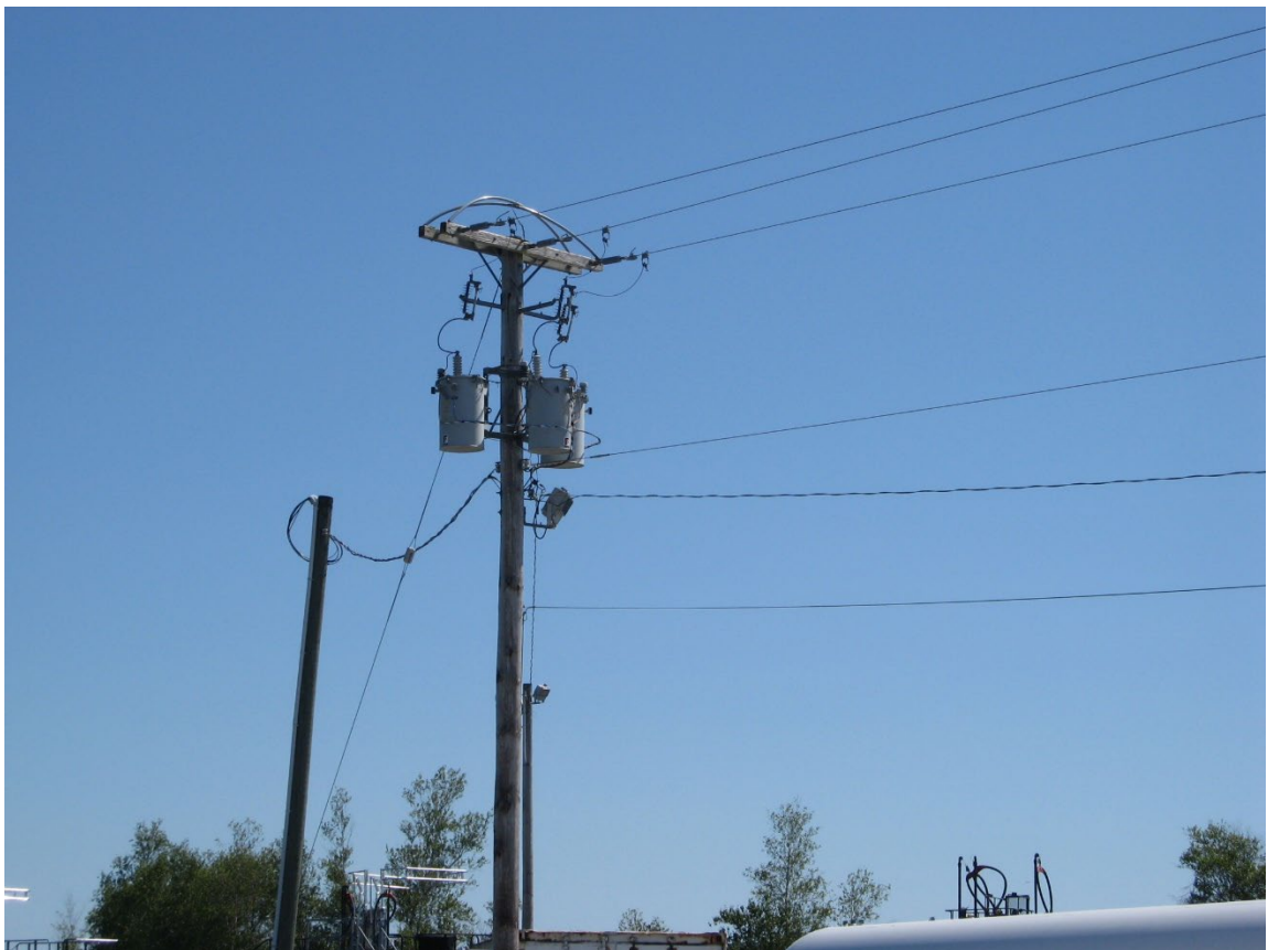
Figure 9: Nest deterrents installed on top of distribution pole
