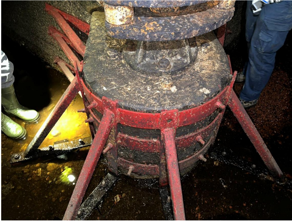
Figure 1: Concrete block supporting quadrant shaft
