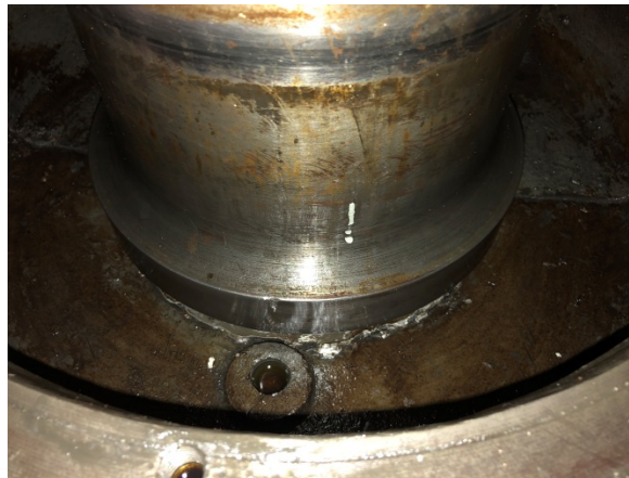
Inside intermediate bearing housing
