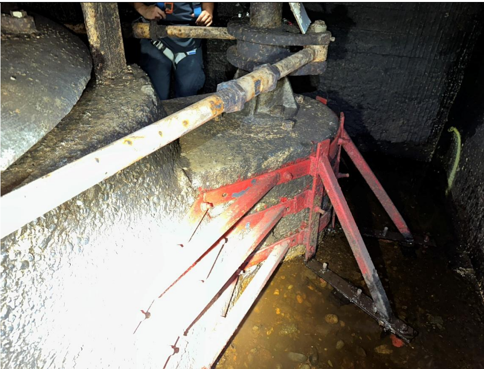
Figure 2: Concrete block supporting quadrant shaft
