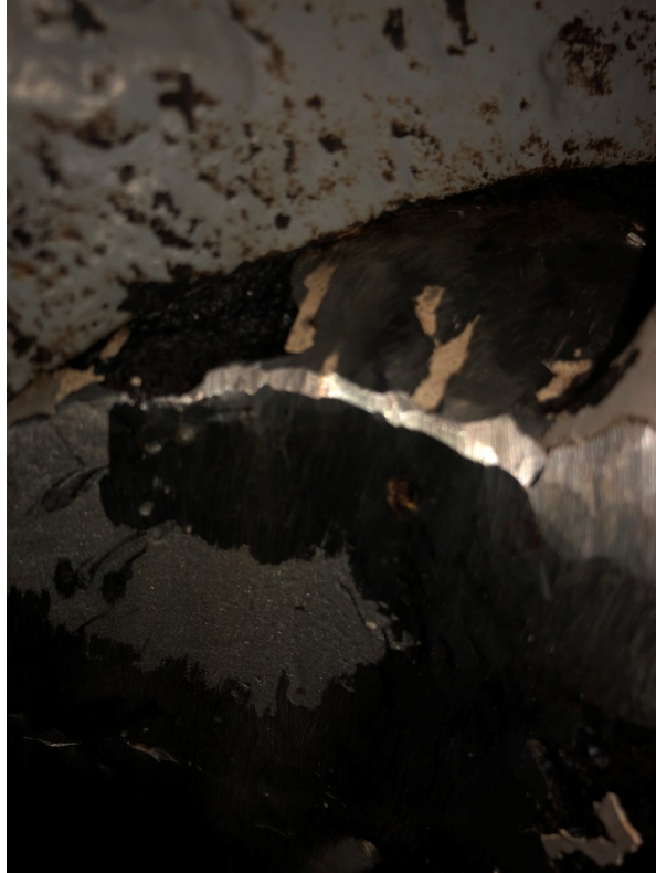
Frosting on stainless, cavitation and rust.
