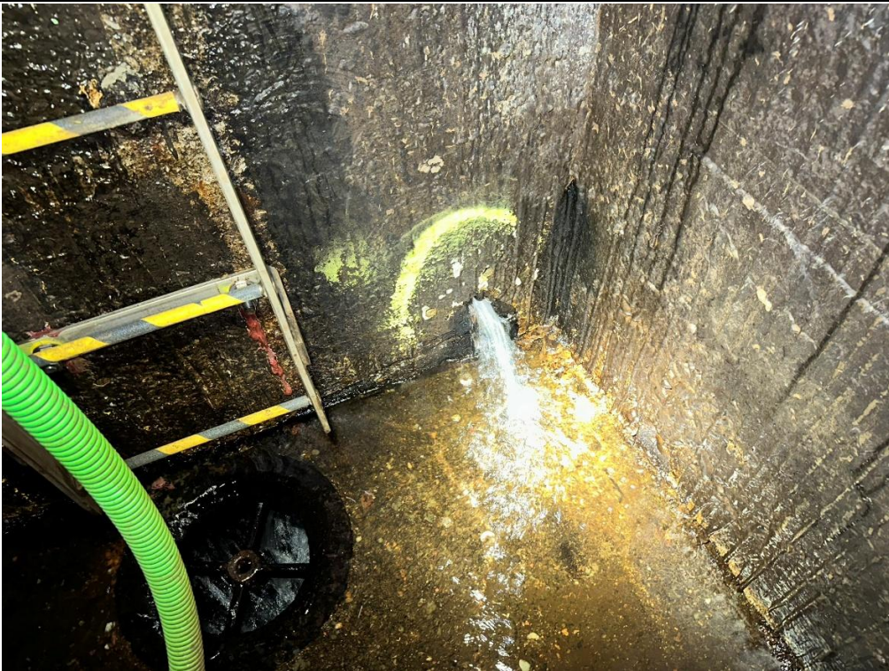
Figure 8: Crack/hole in scroll case wall with water leakage (Corner nearest entrance ladder)
