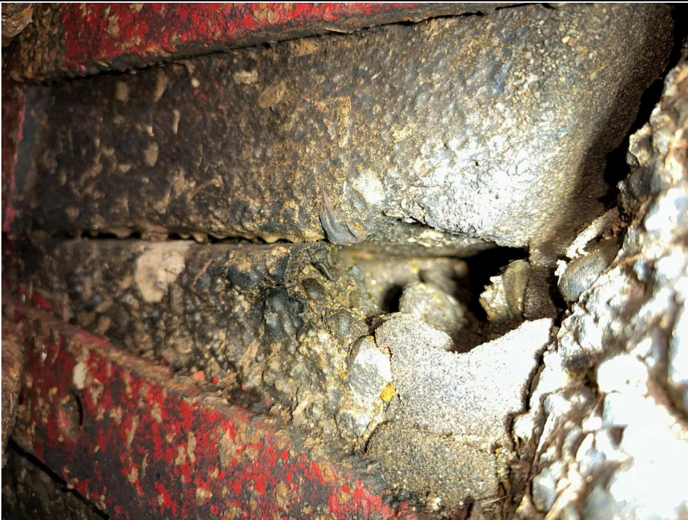
Figure 6: Void in concrete observed on right side of concrete block
