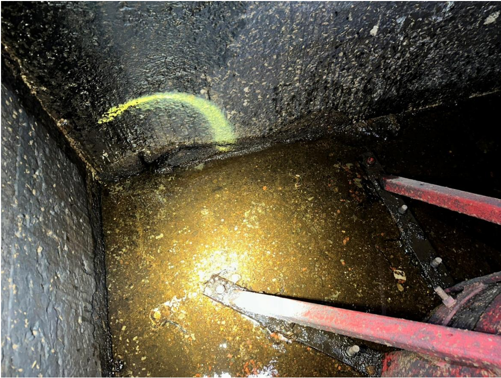
Figure 7: Crack in scroll case wall with water leakage (Corner nearest concrete block supporting quadrant shaft)
