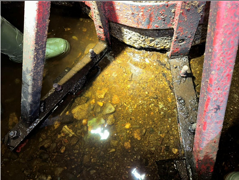
Figure 4: Standing water surrounding concrete block
