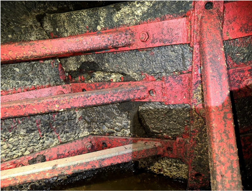
Figure 5: Delaminated/cracked concrete on left side of concrete block
